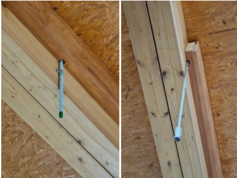
Fig. 9.14 Temperature and humidity sensors in the ceiling of the houses
