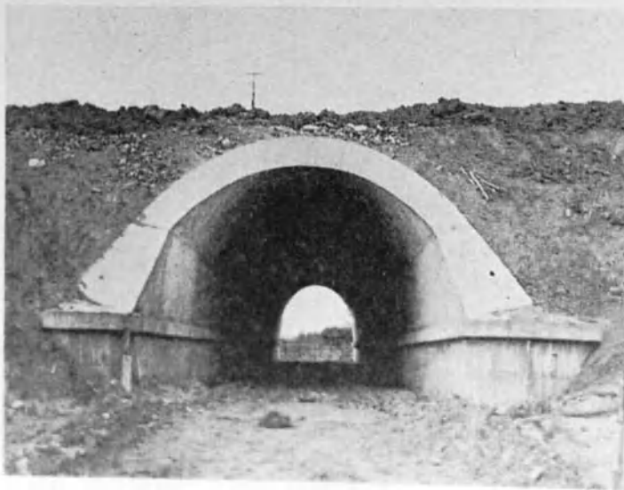
Figure 3.11 Two contrasting underpasses designed by Sir Owen Williams and Partners, from an article by Sylvia Crowe in The Architects' Journal , volume 130, 10 September 1959, p. 160. Reproduced by permission of The Architects' Journal/ Emap Construct.
