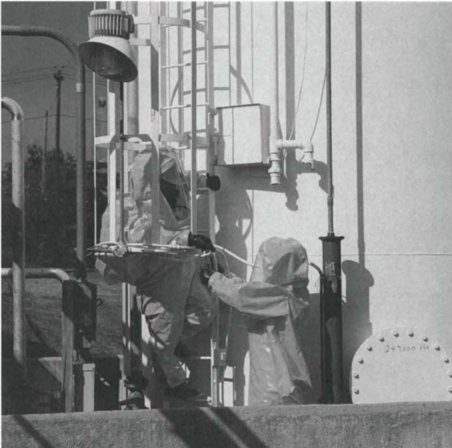
FIGURE 9-3. These two workers appear to be working on a tank farm. One of the workers appears to be descending a caged ladder. Note how his airlines and apparatus are not likely to get tangled in the cage. Photo courtesy of DuPont Tyvek®/ Tychem® protective apparel
