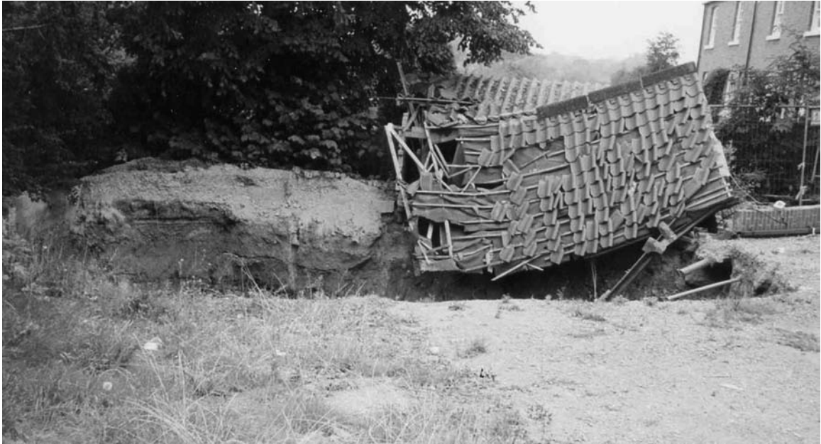
Fig. 8.1 A collapse doline formed in 1997 by failure of the roof of a flooded, natural cave in a bed of gypsum. The collapsed building was a double garage, adjoining a recently constructed detached house on Ure Bank Terrace, Ripon (North Yorkshire, UK). The gypsum bed containing the cave lies within a sequence of dolostone aquifers of Permian age, which are in turn overlain by a major sandstone aquifer of Permian age and permeable river gravels in hydraulic continuity with the River Ure. Vigorous cross-stratal groundwater flow is the root-cause of this dramatic subsidence feature. (Photograph courtesy of Dr John Lamont-Black.)
