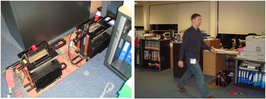
Figure A-35: Active vibration control system in operation: (left) simulating excitation with one shaker while controlling with another and (right) in action reducing floor vibrations induced by walking
