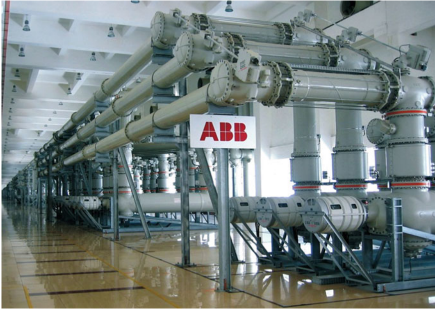
Fig. 4.5 A 550 kV SF 6 gas insulated switchgear installation, at Three Gorges Dam in China with 73 bays (Courtesy of ABB)
