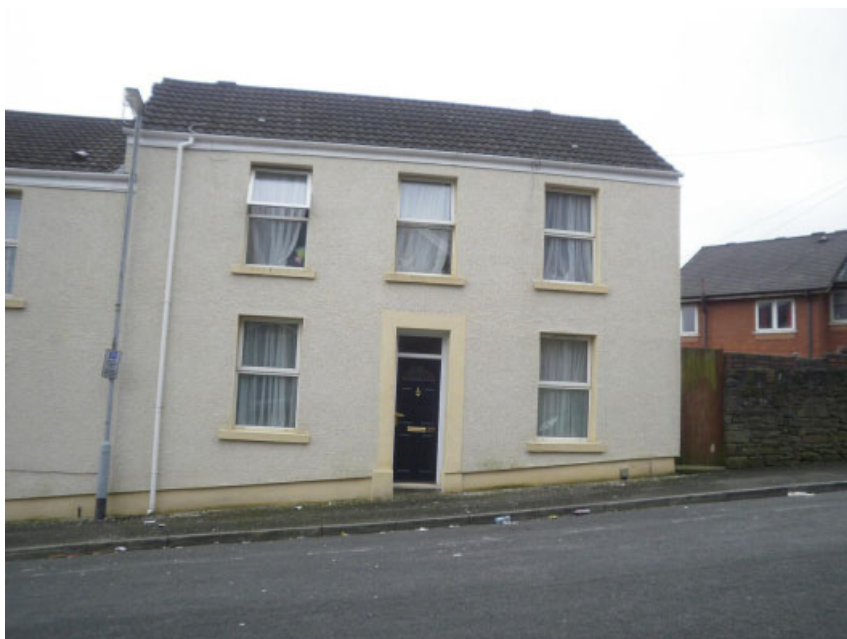
Figure D.9 Photograph of an Arbed case study dwelling after retrofitted EWI was installed.
