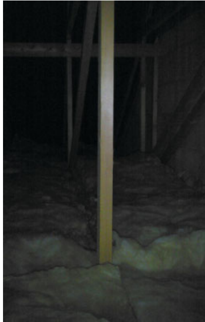
Figure 4.21 Internal visual picture of the roof space with exterior wall and ceiling interface facing the front elevation of the house.
