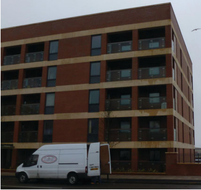
Figure 4.11 External view of the apartment building at practical completion and undergoing occupation (February 2012).
