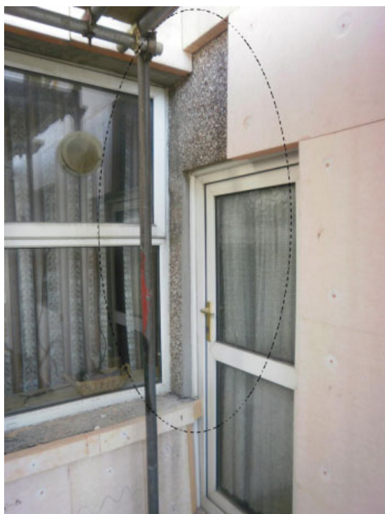
Figure D.3 Example of the lack of a preliminary survey and appropriate technical detail.
