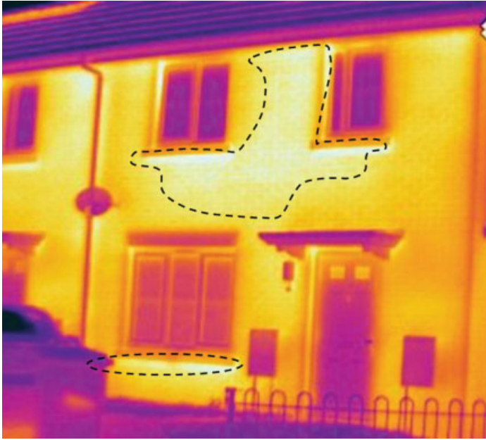
Figure 4.13 External thermogram of the entire house (excluding annex).
