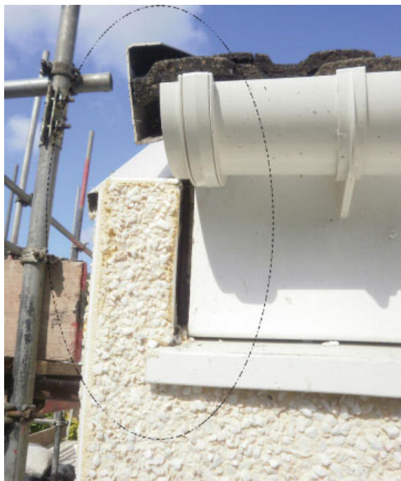
Figure D.2 Example of a poorly planned and executed junction detail.
