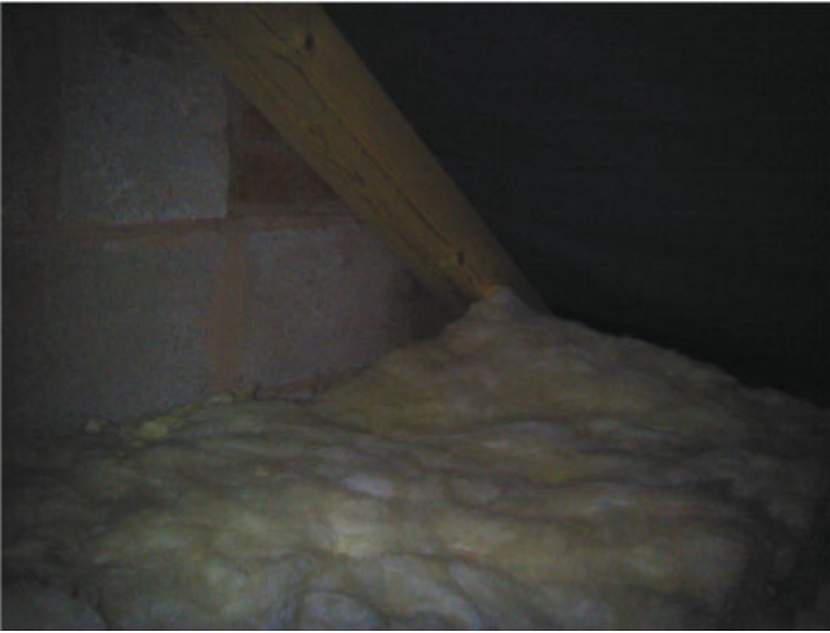
Figure 4.19 Internal view of the roof space with exterior wall and ceiling interface facing the rear elevation of the house.
