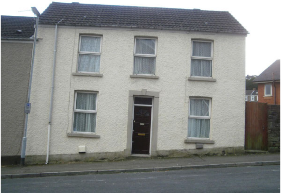
Figure D.7 Photograph of an Arbed case study dwelling before retrofitted EWI was installed.
