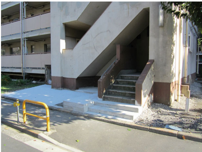
Fig. 7.3 Repaired land subsidence in Tatsumi apartments (Sep. 8, 2011)
