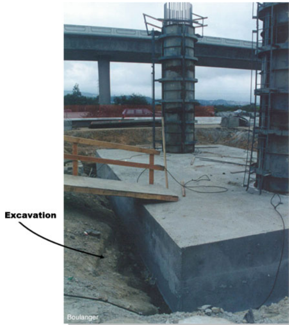
Fig. 21.13 Backfill of the excavation is necessary to provide lateral resistance and stiffness
