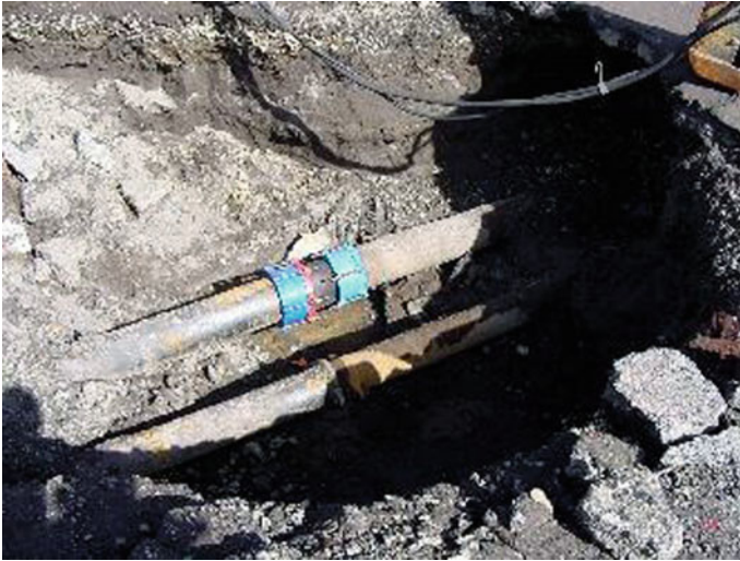
Fig. 7.9 A water pipe broken due to liquefaction
