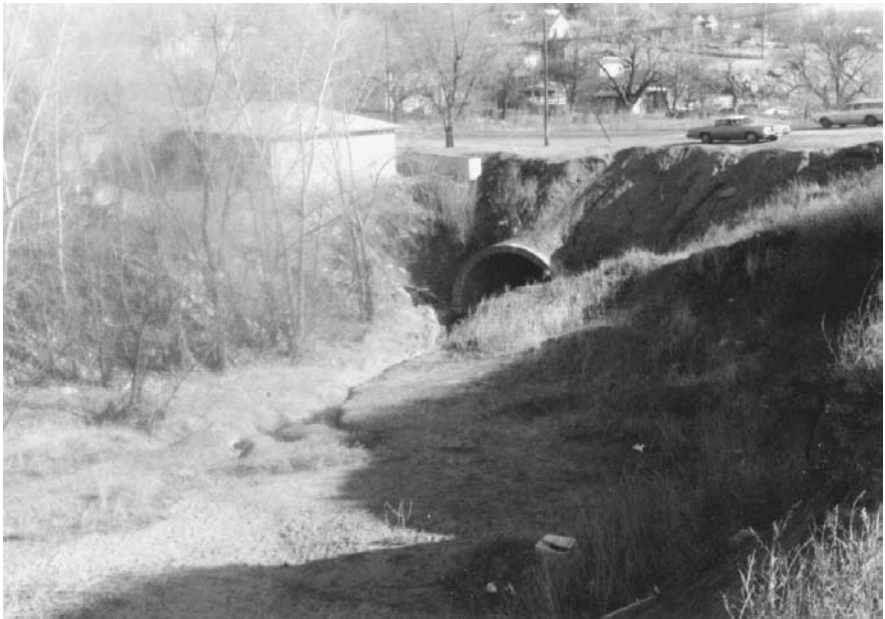
FIGURE 13.7 Partially blocked drain outlet.
