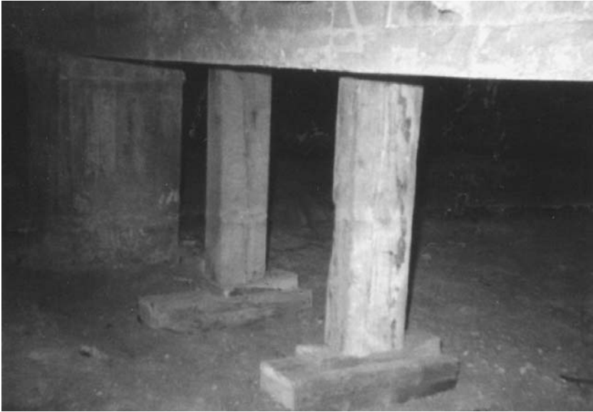
FIGURE 15.2 Timber supports used to correct the missed piers.
