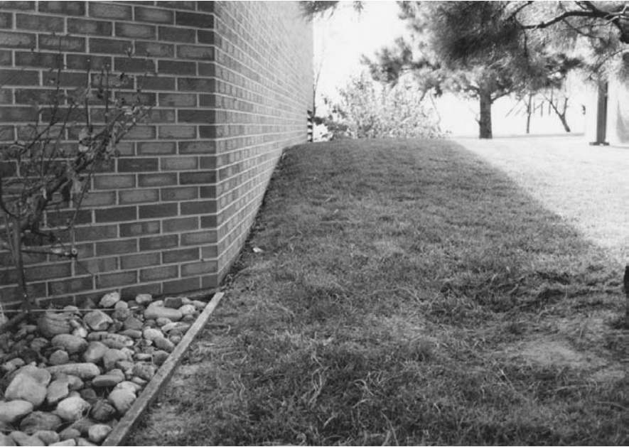
FIGURE 13.8 Cobble above plastic membrane over backfill plank preventing drainage.
