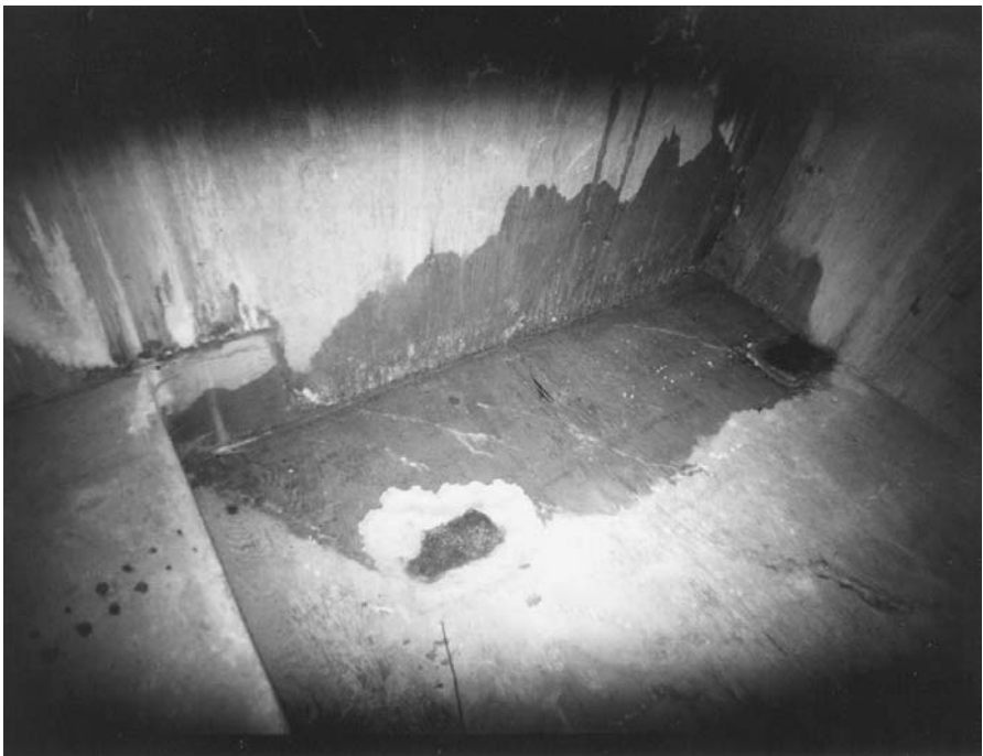
FIGURE 15.1 Water seeped into the lower floor.
