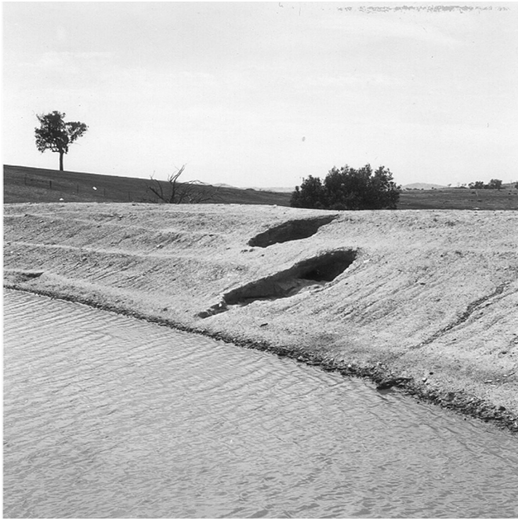
Figure 7.1 Examples of piping failure of a dam constructed of dispersive soils (Soil Conservation Service of NSW).
