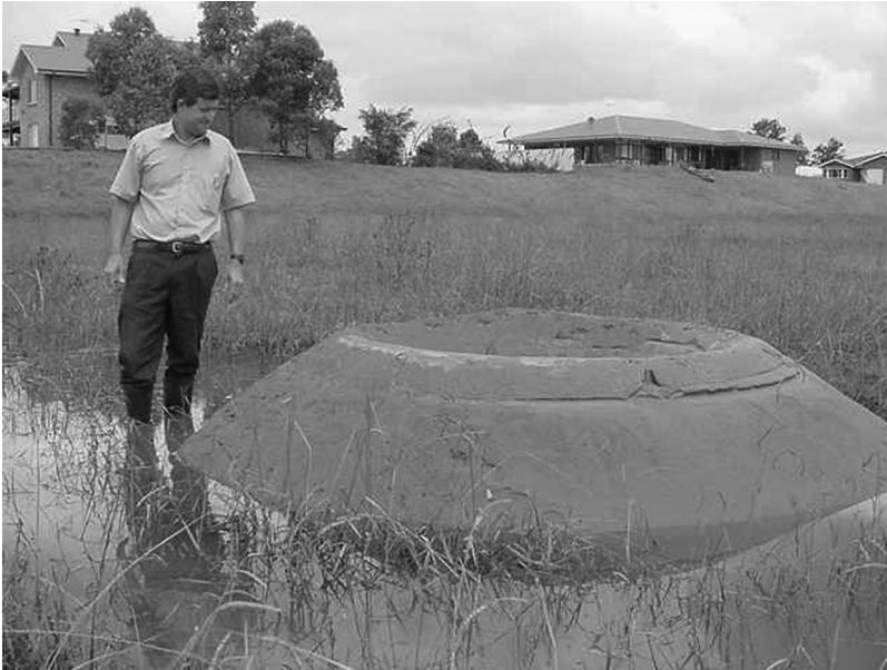
Figure 8.35 Sand boil on the land side of a levee.
