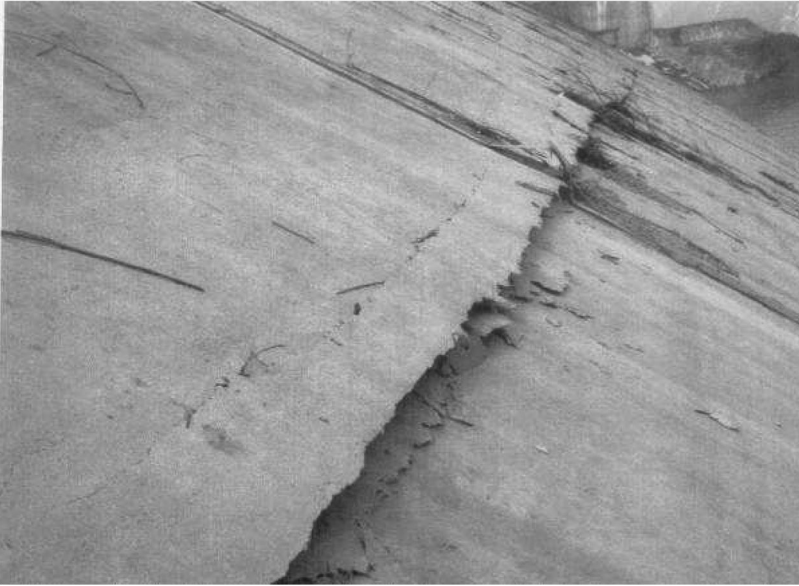
Figure 15.48 Damage of horizontal joint between Stages 2 and 3 of the concrete face of Zipingpu CFRD (Wieland, 2009, photographs courtesy Xu Zeping, China).
