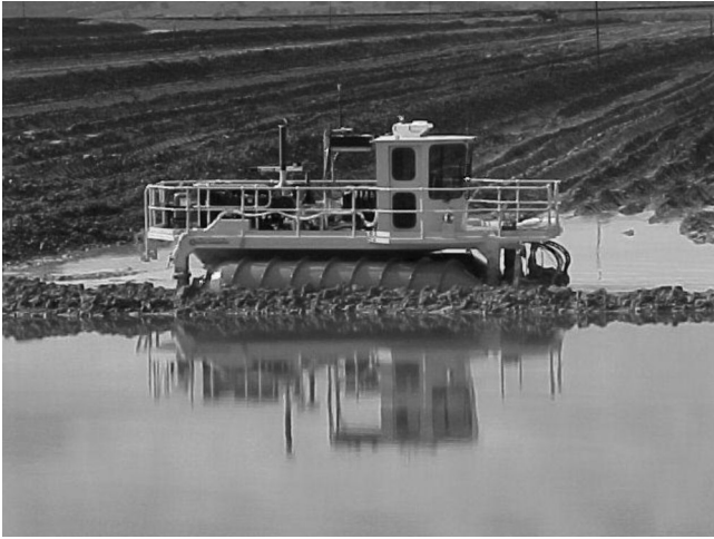
Figure 19.15 Rotating screw device for breaking up the salt layer on top of alumina red mud tailings (photograph courtesy of Geographe Earthmoving).
