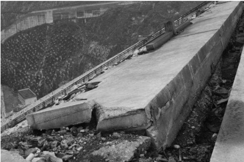
Figure 15.49 Damage at downstream crest of Zipingpu CFRD (Wieland, 2009, photograph courtesy Xu Zeping, China).
