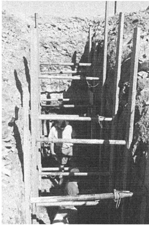
Figure 5.11 Timber supported trench/pit in Happy Valley Dam, Adelaide, South Australia (courtesy SMEC and SA Water).
