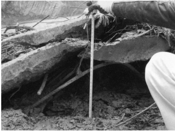
Figure 15.20 Campos Novos Dam. Central compressive vertical joint failure (Cruz et al. , 2009).
