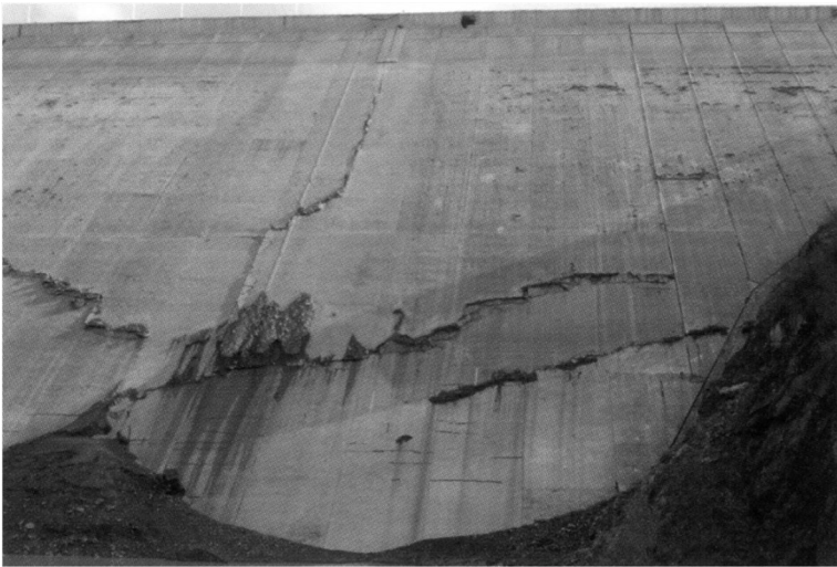
Figure 15.45 Campos Novos Dam face slab failure (Cruz et al. , 2009).
