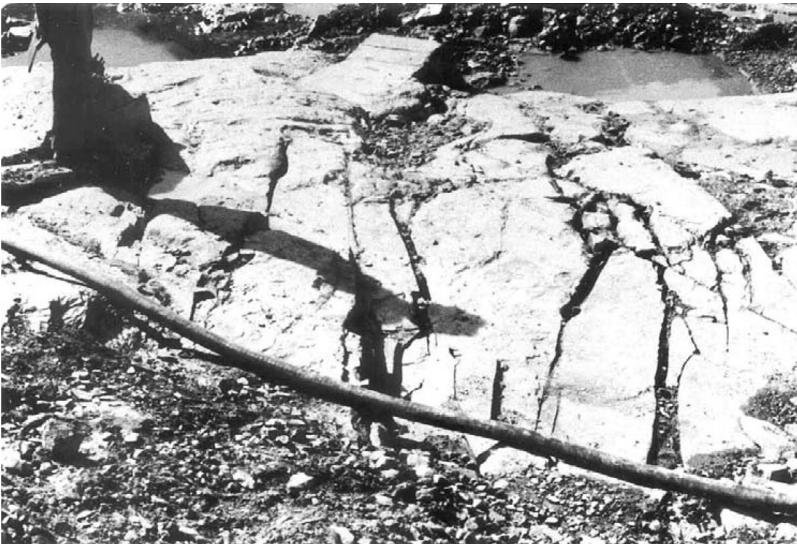
Figure 2.9 Upper surface of Unit E sandstone at Mangrove Creek Dam valley bulge, showing joints open as much as 100 mm, clay-filled in part.
