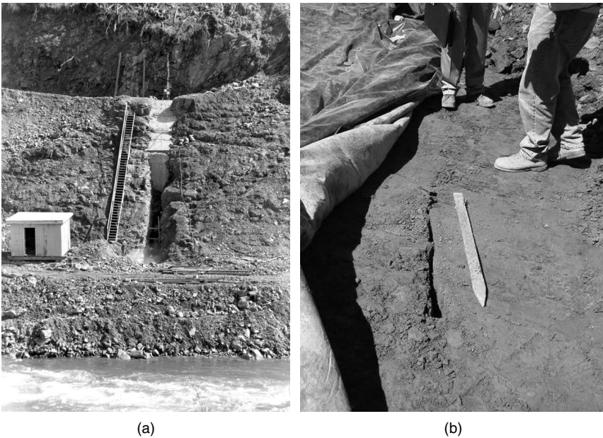
Figure 8.13 Buffalo Dam. (a) Bench in the abutment over which transverse cracking occurred and (b) Transverse crack (Courtesy of Goulburn-Murray Water and URS Australia).
