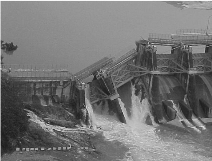
Figure 16.30 Damage to Shikang dam in Taiwan in 1999. The vertical displacement was about 9 m and the horizontal displacement was about 1.5 m into the abutment.
