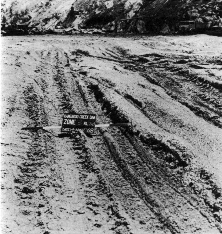
Figure 3.15 Slurry (Gravelly sandy silt) formed on the top of schist rockfill layer as a result of weathering and compaction by 4 passes of a 10-tonne vibrating roller (Trudinger, 1973).
