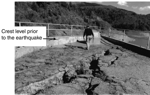
Figure 8.22 Transverse and longitudinal cracking of Austrian Dam during the Loma Prieta earthquake: (a) Plan of the cracking. (b) Cracking adjacent to the spillway. (Forster and McDonald, 1998, Photograph courtesy of S. Todaro).
