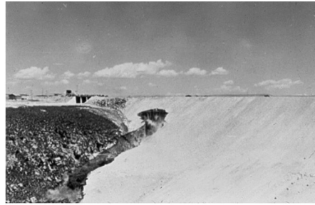
(b) Concentrated leak and pipe at 11:30 am
