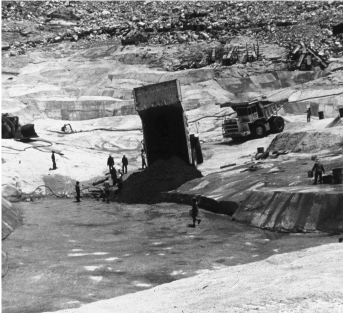
Figure 17.4 Dental concrete in the cutoff at Kenyir Dam (courtesy of Snowy Mountains Engineering Corporation).
