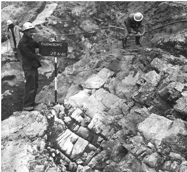
Figure 17.7 Application of pneumatically applied mortar on seams in the cutoff foundation of Blowering Dam (courtesy of Snowy Hydro).
