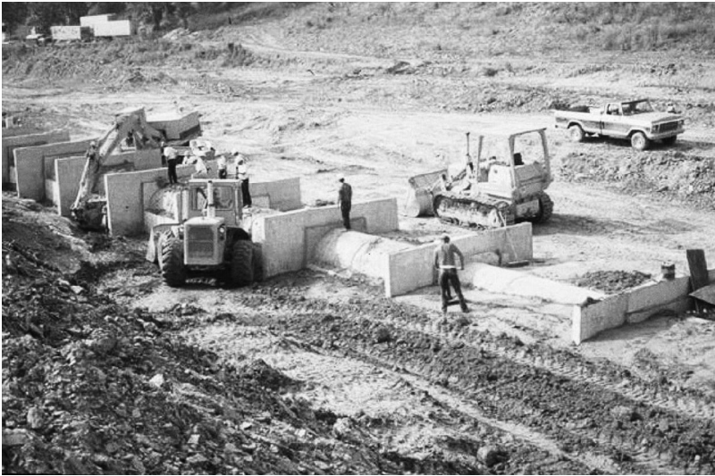
Figure A3.1 Example of poor detailing of seepage collars around a conduit (from FEMA 2005).
