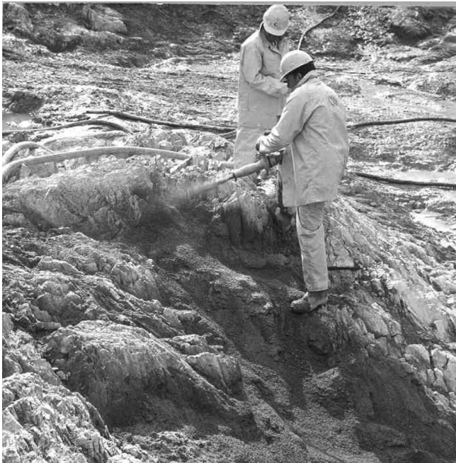
Figure 17.6 Cutoff foundation for Blowering Dam showing open joints being treated with pneumatically applied mortar, but no treatment for other joints (courtesy of Snowy Hydro).
