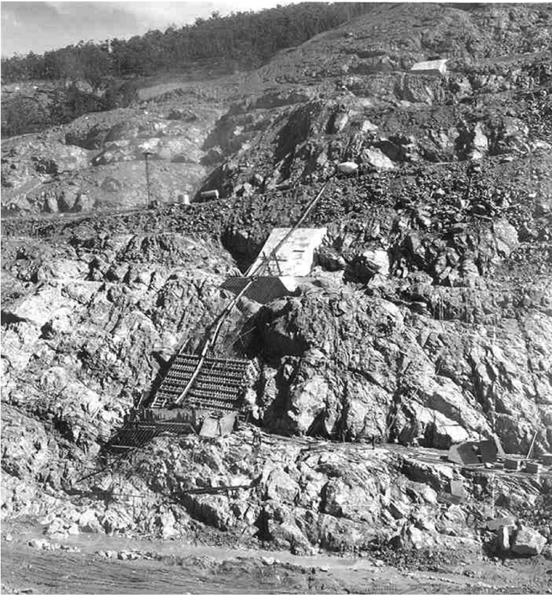
Figure 17.3 Abutment of Dartmouth Dam showing cleanup in cutoff foundation, and construction of the grout cap (courtesy of Goulburn-Murray Water).
