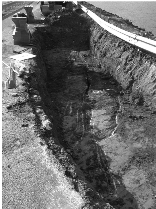
Figure 11.12 Cracking and softening due to settlement and lateral spreading at the crest of an embankment dam (Courtesy Goulburn Murray Water and URS Corporation).
