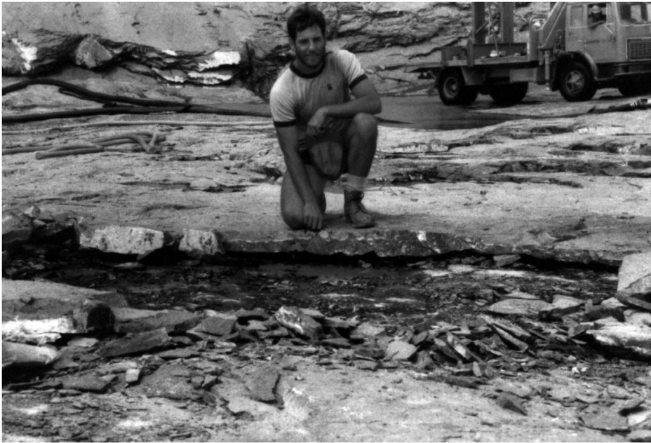
Figure 17.28 Slab of rock which has lifted about 50 mm due to stress relief. Monolith LHZ adjoining to LHI (photograph courtesy of SunWater).
