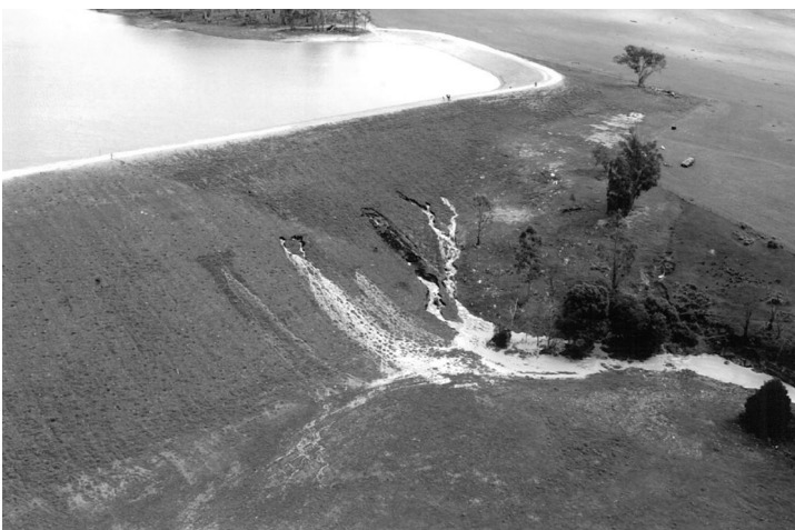
Figure 8.18 Concentrated leaks in Tunbridge dam possibly related to collapse settlement of a poorly compacted layer.
