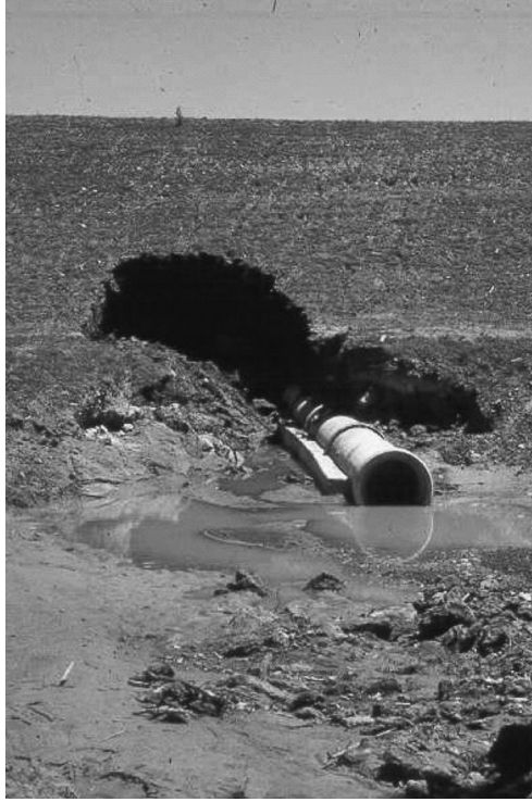
Figure 13.12 Piping failure of a dam around the outlet conduit.
