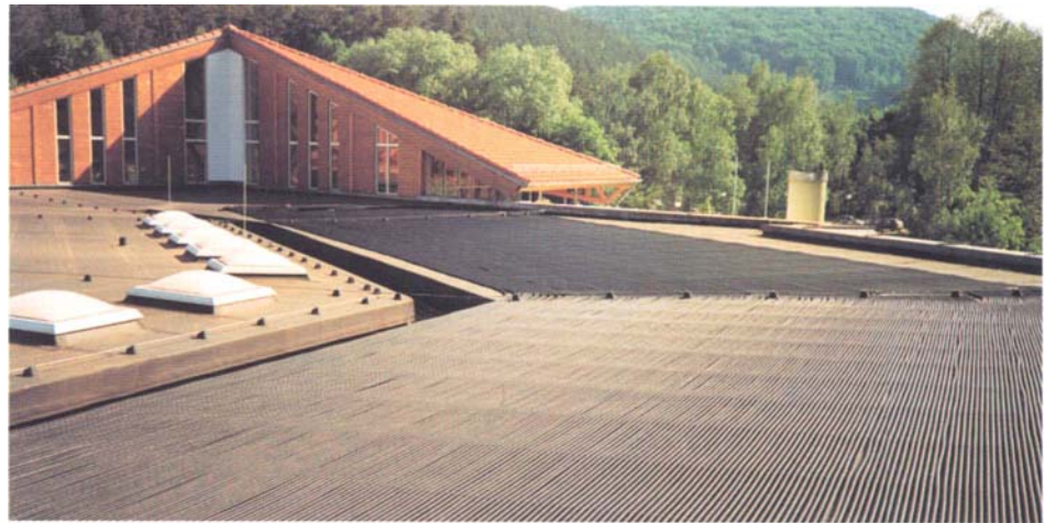
Figure 7.1. Solar absorber in an open-air pool. Source: Lange GmbH, Telgte
