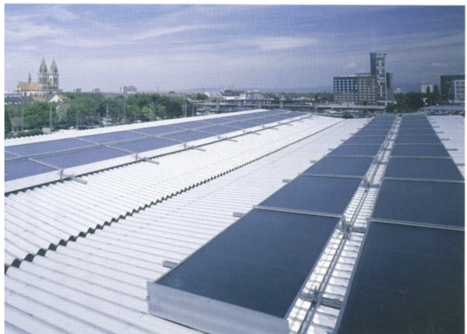
Figure 9.1. 100 m 2 collector system for a solar-powered air-conditioning system in Freiburg, Germany. Source: Fraunhofer ISE
