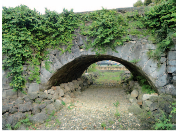
Fig. 10.9 San Antonio Bridge, Hagatña, Guam. (Courtesy of the US National Park Service)
