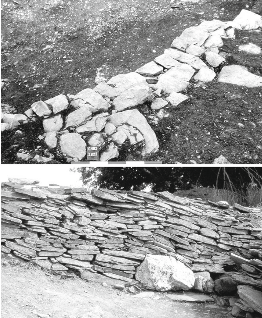
Fig. 12.18 Top : wall 2823 from above showing its revetting in situ upper fill of ditch 4079, with the surface of cut 2826 beyond. Bottom : detail of wall 2823 showing use of quartz blocks at base and drystone construction
