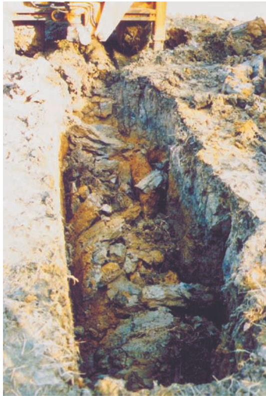
Figure 1.8 Pit collapse immediately after removal of shoring.
