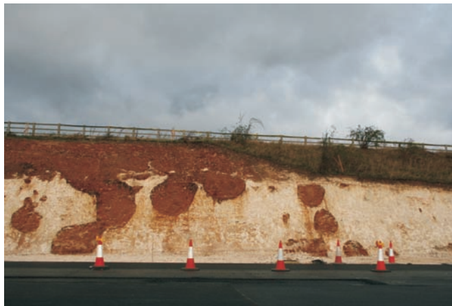
Figure 10.5 Infilled dissolution features in chalk road cutting showing the complex geometry of such features (photograph courtesy of Digby Harman).
