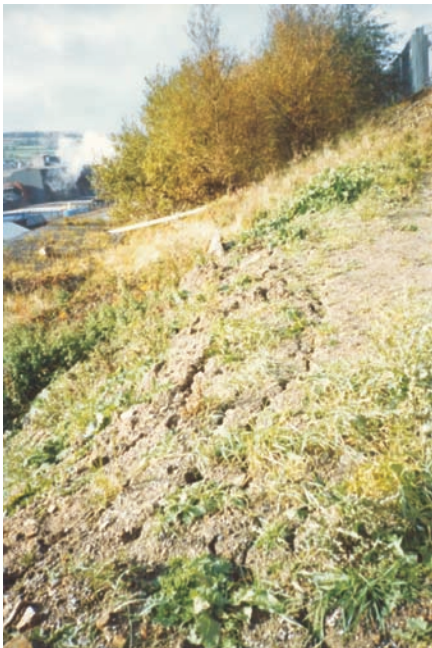
Figure 1.2 Engineering works example – slope instability.
