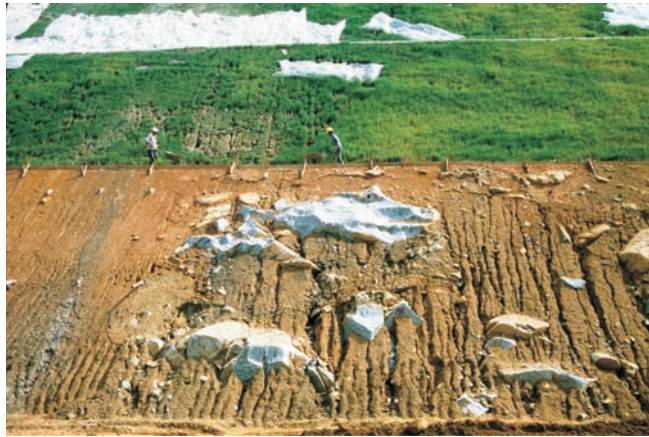
Figure 2.1 Corestones of relatively fresh rock material within completely weathered material in Hong Kong as envisaged by the column 2 approach in Table 2.5 (photograph courtesy of Steve Hencher).
