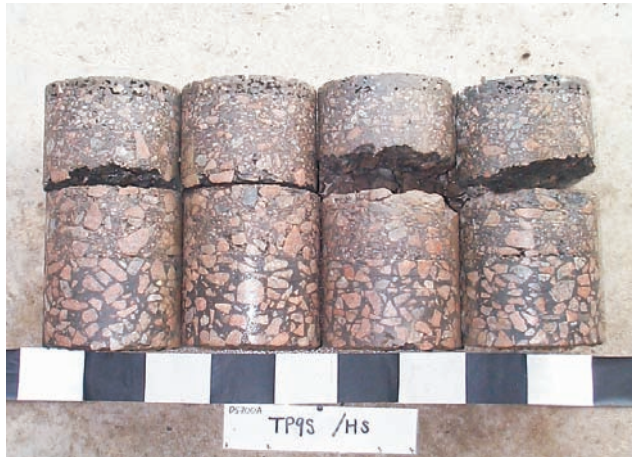
Figure 14.5 Cores of asphalt concrete of a flexible road pavement showing multiple construction layers (photograph courtesy of Soil Mechanics).
