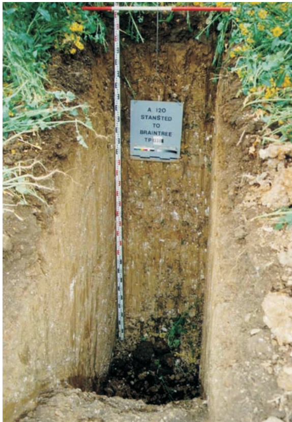
Figure 16.7 Trial pit record photo with good lighting and scale and visibility to the base of the pit (photograph courtesy of Soil Mechanics).
