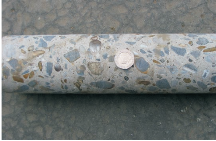
Figure 14.4 Core of cement concrete showing reinforcement steel to either side of the coin.
