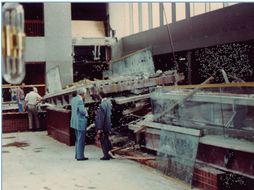
Fig. 3.1 Hyatt regency walkways following collapse (Wikipedia Commons 2013 )
