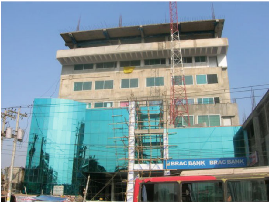
Fig. 3.6 Rana Plaza factory building before collapse (Wikipedia Commons 2013)
