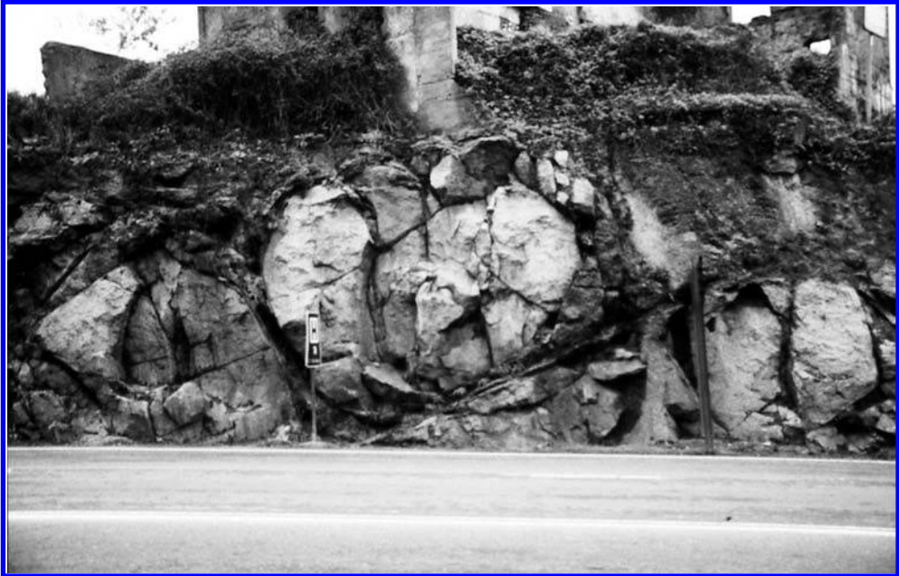
Figure 5.13. Shear planes with conjugate system of discontinuities and corestones exposed in road cutting at A Coruña, Galicia, NW Spain.
