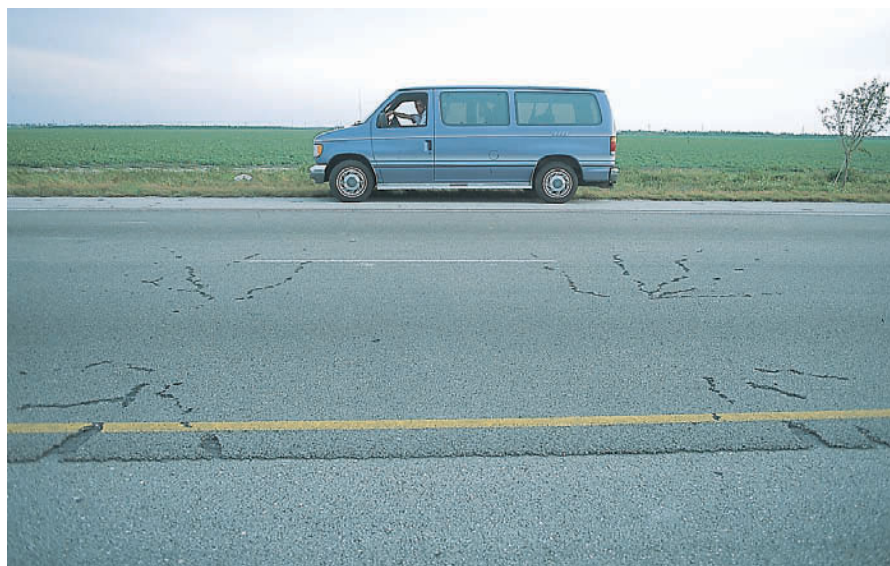
■ FIGURE 10.25 The four marks on the road surface represent areas where lightning, after striking a car traveling along south Florida's Sunshine State Parkway, entered the roadway through the tires. Lightning flattened three of the car's tires and slightly damaged the radio antenna. The driver and a six-year-old passenger were taken to a nearby hospital, treated for shock, and released.
