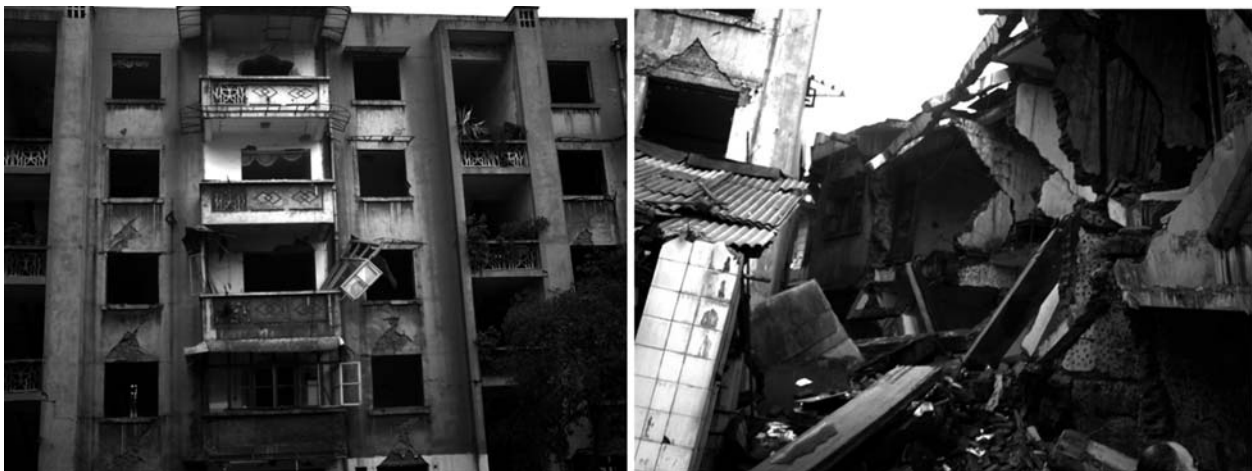
Figure 4-3. Concrete structures with many walls stands well (left) and totally collapsed brick wall structures
