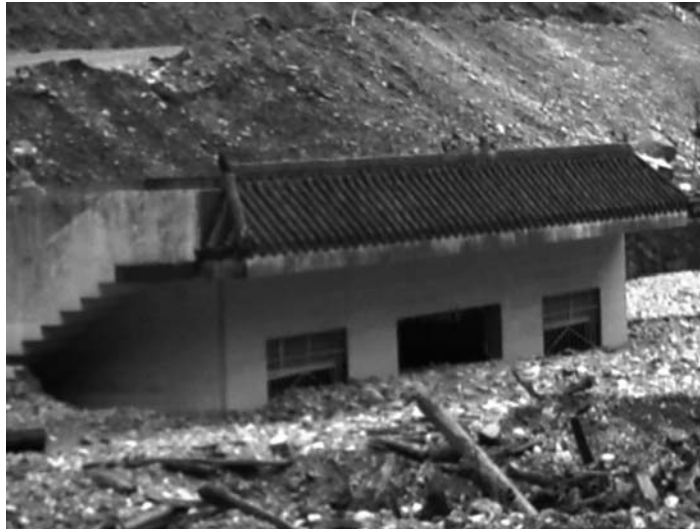
Figure 4-2. A house damaged and buried during landslides
