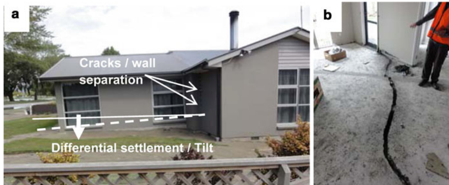
Fig. 1.11 Observed typical liquefaction-damage to house foundations: (a) differential settlement resulting in tilt and damage to house; (b) large crack in a concrete slab
