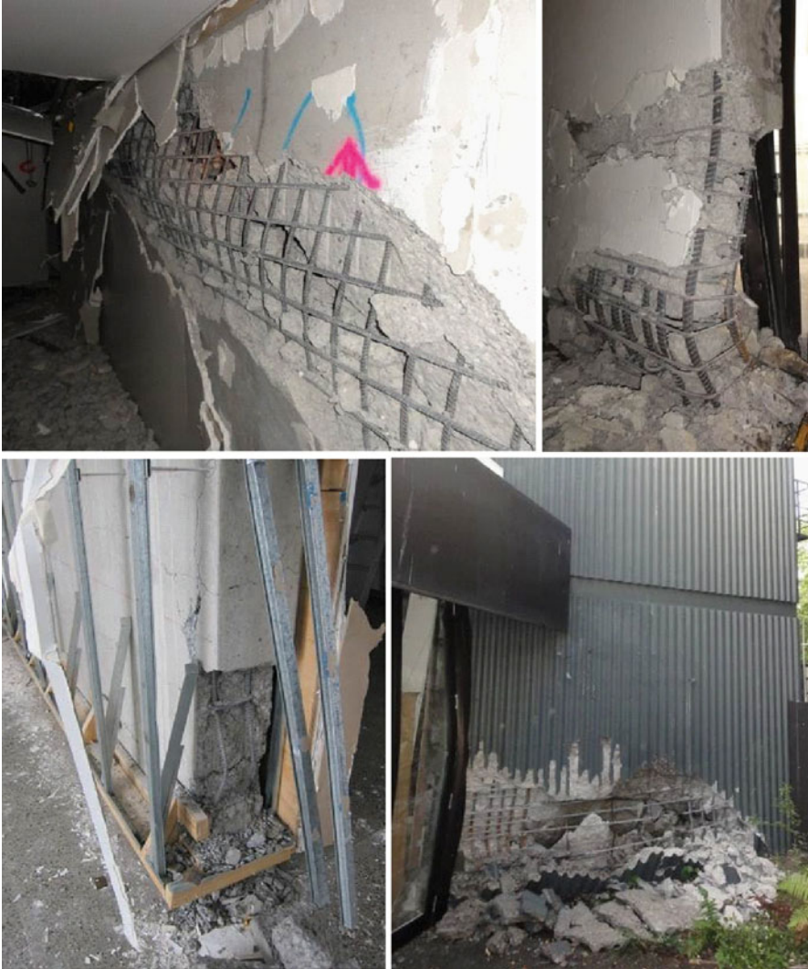
Fig. 1.22 Damage and failure mechanisms of shear walls in modern multi-storey buildings (From Kam and Pampanin 2011; Kam et al. 2011)
