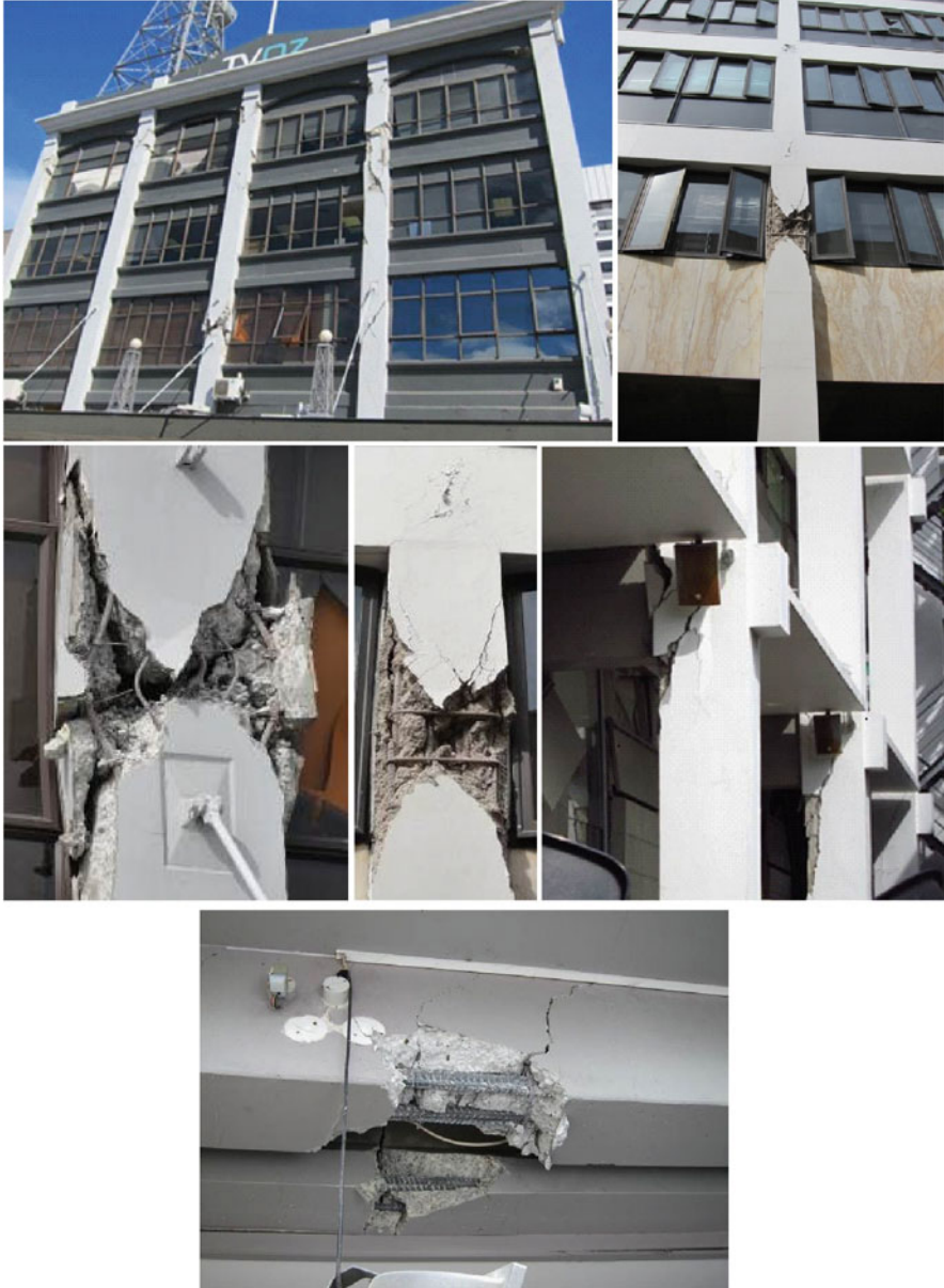
Fig. 1.20 Example of damage and failure mechanisms in pre-1970 Reinforced Concrete frame buildings: column and joint shear failure, “captive” column, beam lap splice failure (From Kam and Pampanin 2011; Kam et al. 2011)
