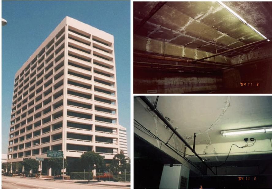
Fig. 7.5 Damage to the 13 story Sherman Oaks building during the 1994 Northridge earthquake
