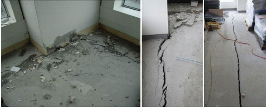
Fig. 1.24 Extensive damage of floor diaphragm and loss of floor support due to the beam-elongation effects of concrete frame inelastic response
