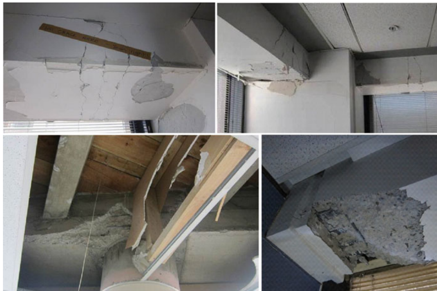
Fig. 1.21 Typical beam plastic hinge mechanism and damage in modern (post-1970s) reinforced concrete moment-resisting frame buildings (From Kam and Pampanin 2011; Kam et al. 2011)
