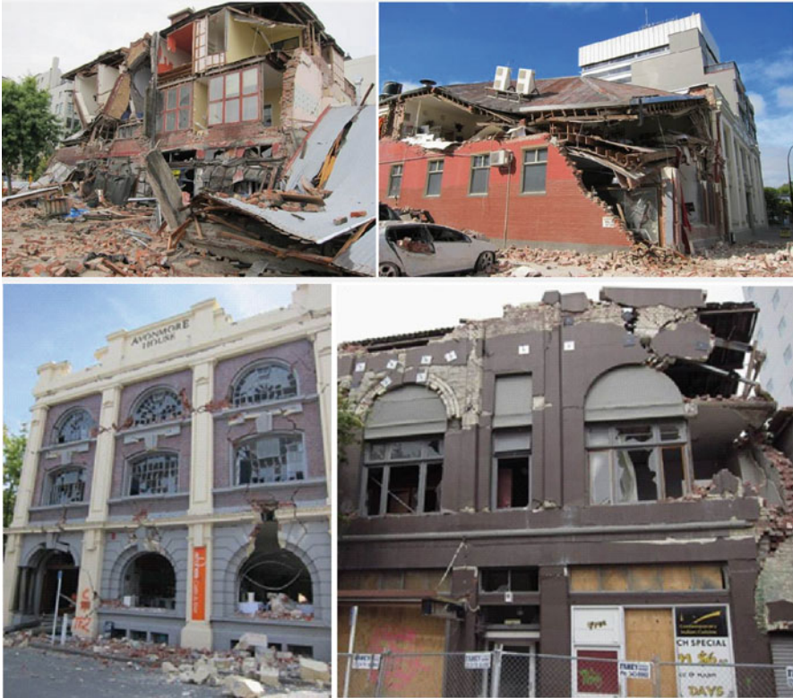
Fig. 1.19 Example of damage and failure mechanisms in unreinforced masonry buildings (From Kam and Pampanin 2011; Kam et al. 2011)
