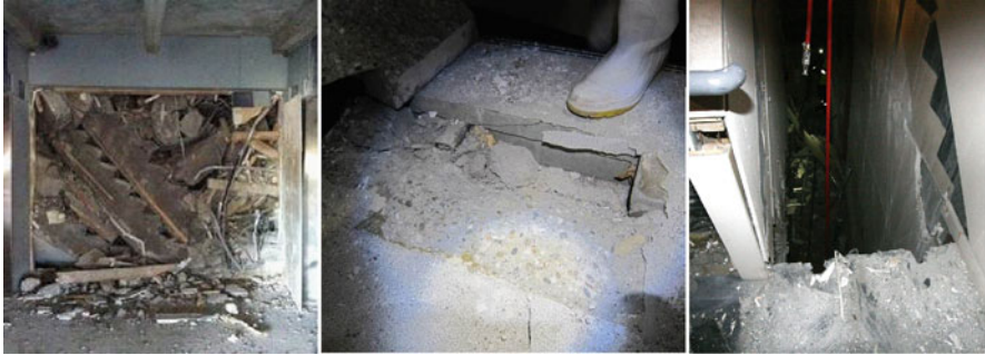
Fig. 1.23 Collapse and damage of stair systems in multi-story buildings (From Kam and Pampanin 2011; Kam et al. 2011)
