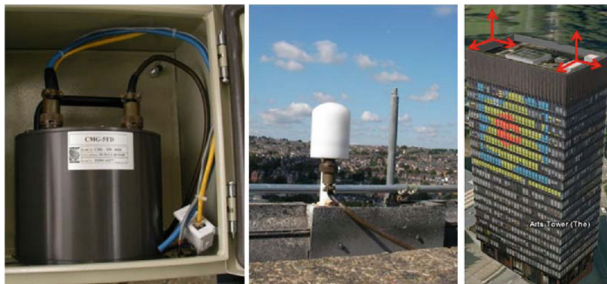
Fig. 6.5 Triaxial accelerometers and GPS antennae for FSDL system
