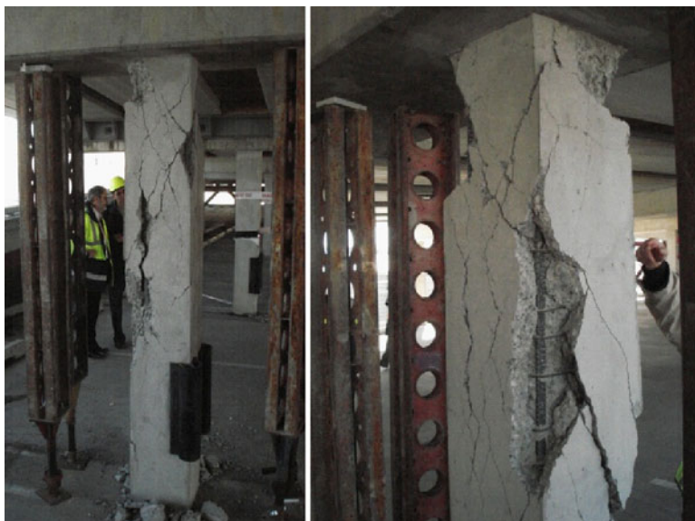
Fig. 1.25 Severe damage with loss of vertical load-bearing capacity in columns with inadequate transverse reinforcement as part of the “gravity-load systems” due to displacement compatibility with the lateral load resisting systems
