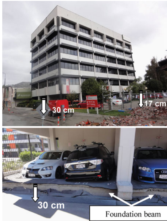
Fig. 1.14 Building on pile foundations in area of severe liquefaction showing large settlements of the surrounding soils relative to the foundation beams
