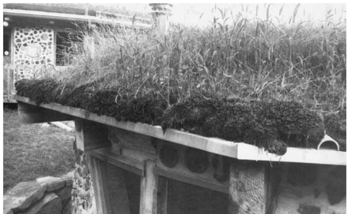
Fig. 8.18: Moss sods drain well, retain the earth and look natural. Note "half-pipe" for drainage.
