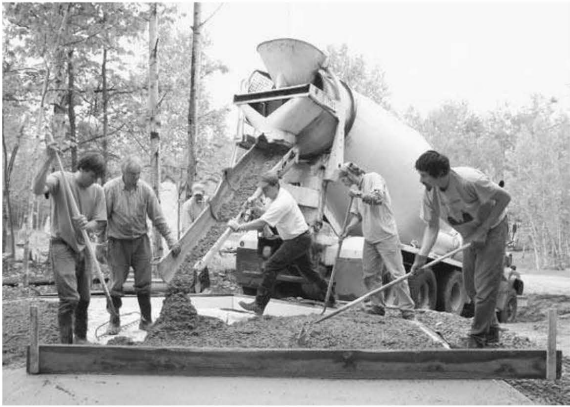
Fig. 3.7: EARTHWOOD: LAYING OUT AND DIGGING THE FOOTING TRACKS A crew of six made easy work of pouring the small four-cubic-yard monolithic floating slab at the new octagonal guesthouse at Earthwood.
