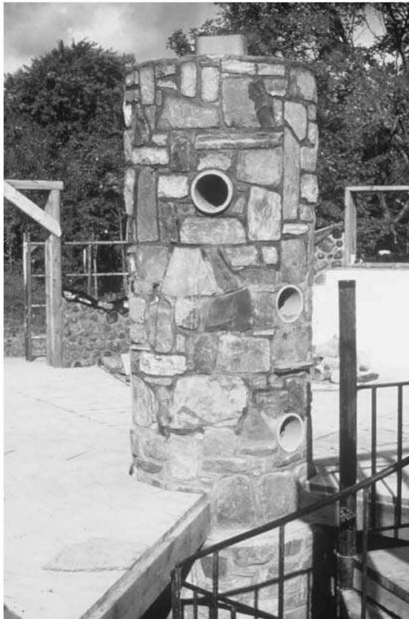
Fig. 10.3: The masonry stove at Earthwood.
