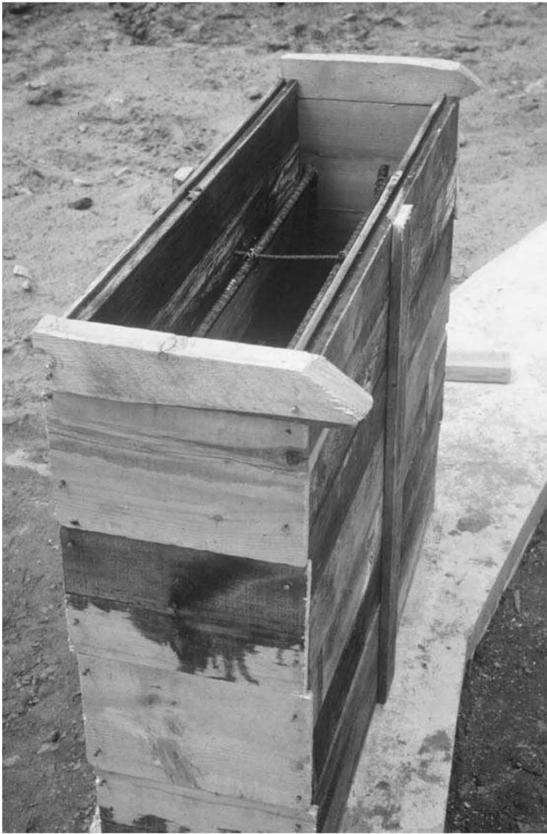
Fig. 4.16: We formed the buttresses with recycled 2 × 6" tongue-and-groove silo boards. of the sand to slow the set. And (3) Specify two trucks, maybe 45 minutes apart, so that there is no waiting for the second half of a large pour.
