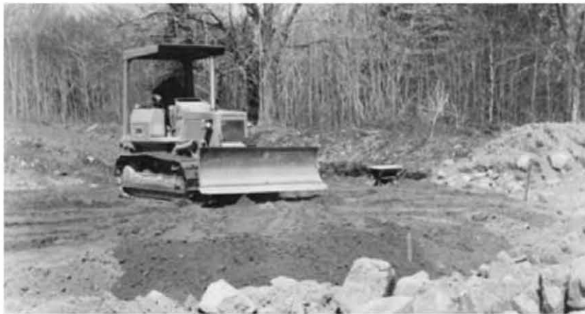
Fig. 3.5: Three or four runs of sand are built up and individually compacted, resulting in a final compacted pad of at least 18".
