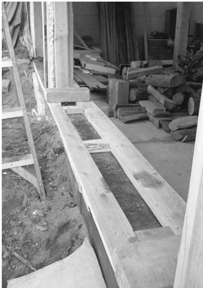
Fig. 12.2: The poured wall is broadened to accommodate the 16-inch cordwood wall by the use of this 2 × 6" detail, described in the text.
