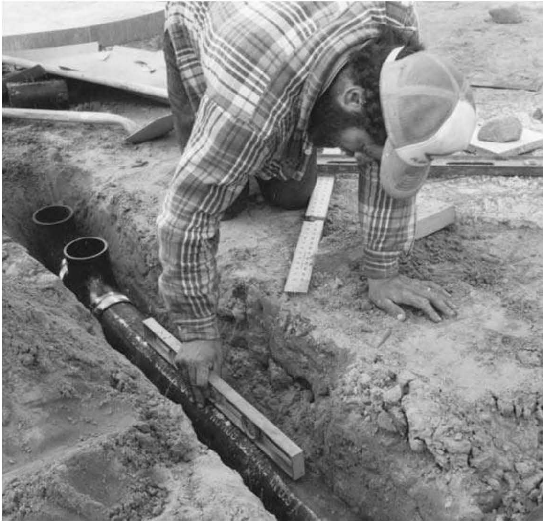
Fig. 4.10: Installation Tips for Underfloor Plumbing Dennis Lee Plan the plumbing so that all traps are accessible. In the case of a bathtub or shower on the first floor, this will usually necessitate “boxing out” a small area so that concrete cannot get in around the trap or drain. An 18-inch square box made of 2-by-6 material can be seen in Figure 4.9. It provides access to our shower drain and trap. Another good reason for the box is that – thanks to the ubiquitous Mr. Murphy of the famous law – it is very difficult to get the drain in exactly the right place with respect to adjacent walls, which are still non-existent at this point in time. Within the box, you can still make final adjustments to a drain location at the time of shower- or tub-base installation.
