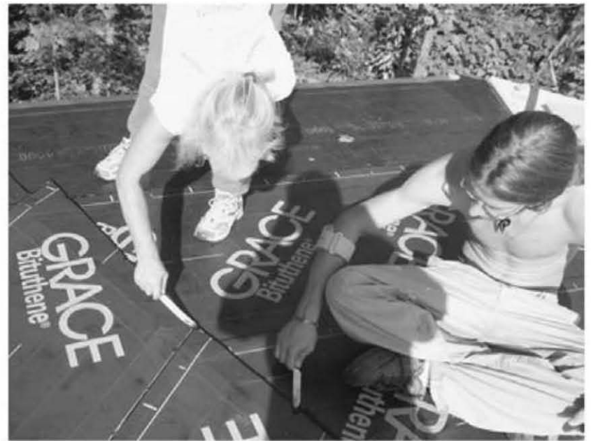
Fig. 8.3 (above): Jaki and Darin Roy feather the edge of the mastic with pointing knives, to approximate the factory edge of the Bituthene® membrane. The mastic stops the cut edge from raising up or "fish-mouthing."
