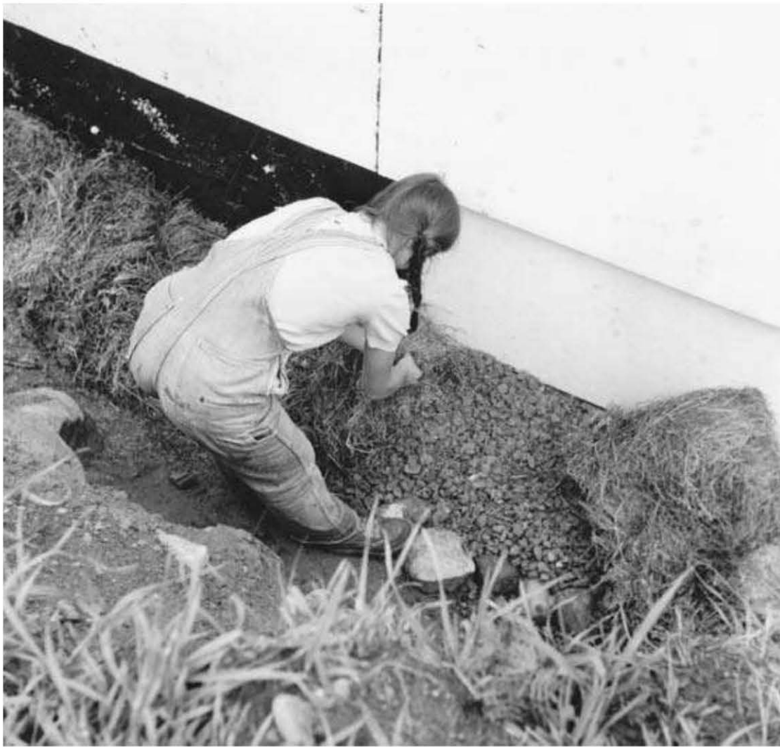
Fig. 7.15: Jaki spreads hay or straw on the crushed stone surrounding the drainage tubing.
