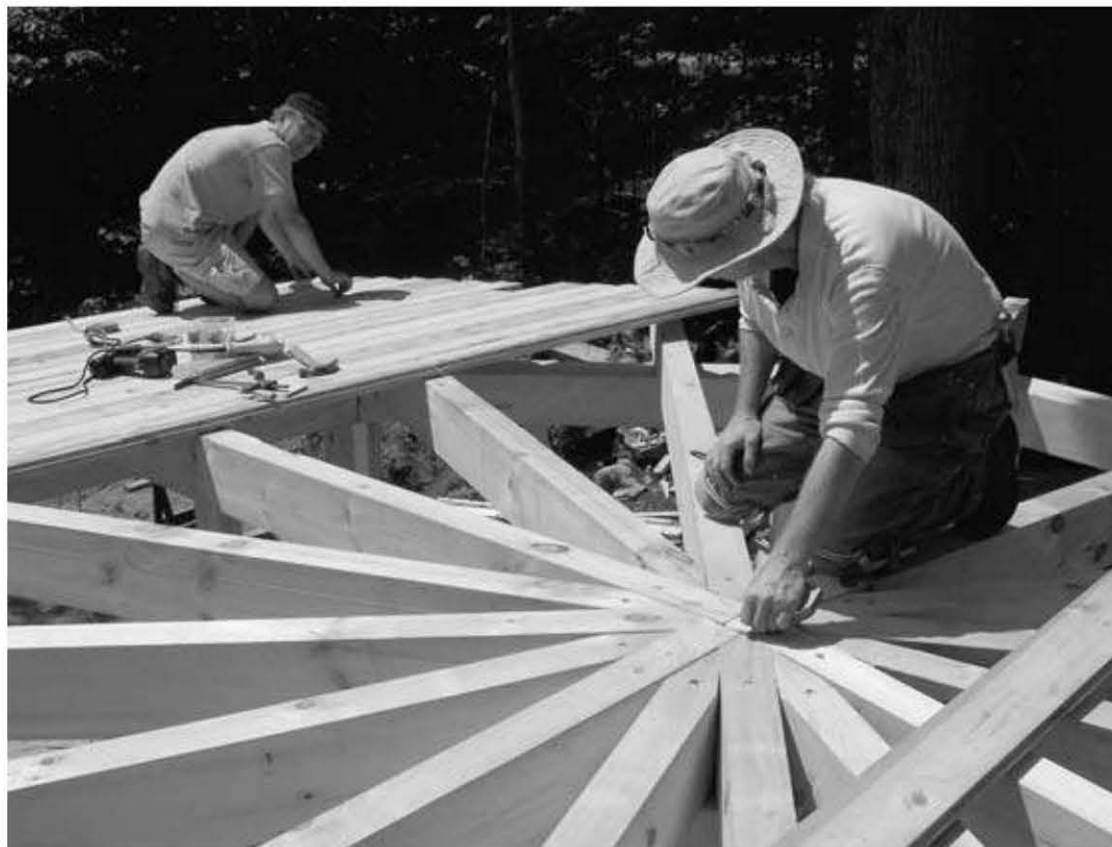
Fig. 6.18: Planking the roof at the Stoneview guesthouse was a lot like doing the Earthwood roof. Here, we snap a line on the planks, but directly over the middle of the 4 × 8" rafters. Next we cut off all the "waste" at once with a circular saw.
