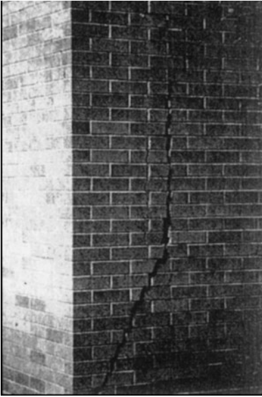
FIGURE 9.28 Stair-step cracking in a masonry wall due to differential settlement [9.19].
