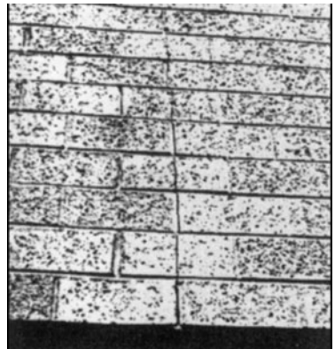
FIGURE 9.27 Cracking in masonry wall due to excessive deflection of supporting beam or lintel [9.18].
