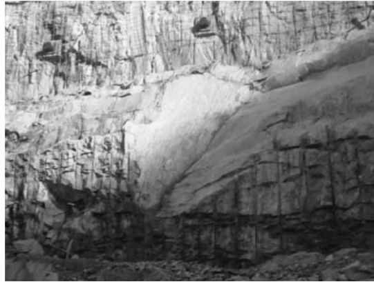
Figure A14 Rock wedge sliding at rock anchor beam.
