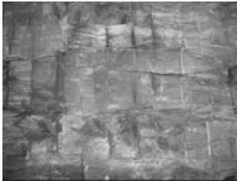
Figure A11 Tensile cracking at the erection bay sidewall.
