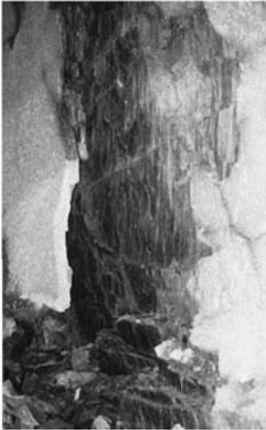
d Sprayed concrete spalling
