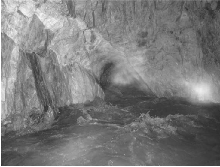
Figure 6.76 High pressure flow point at lower sidewall near AK14+760 in Access Tunnel #A (HydroChina Huadong Engineering Corporation, 2005).
