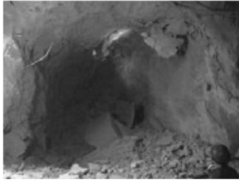
Figure A8 Strong fault rockburst in the bus tunnel.
