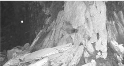
a Spraved concrete and surrounding rock collapse
