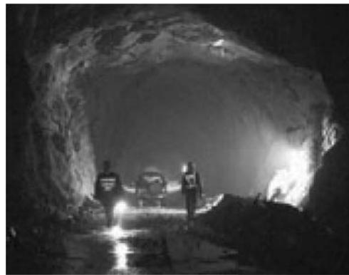
Figure A9 V-shape failure in auxiliary tunnel.
