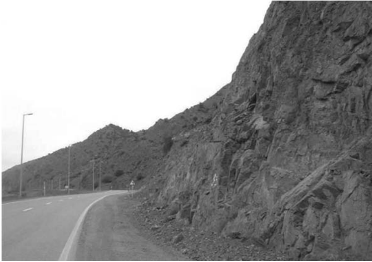
Figure 3.41 Example of the roadside rock mass along the Khosh-Yeylagh Main Road in a mountainous area approximately 90 km north of Shahrood City, north-eastern Iran (from Naghadehi et al. , 2011).
