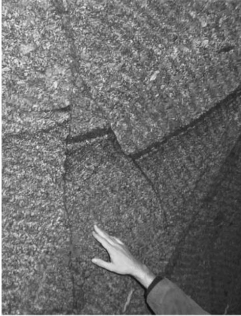
Exposure 15. Machine excavated tunnel sidewall in the granitic Bohemian Massif, Czech Republic
