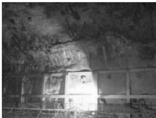
Figure A24 Fracture zone bulging outward at powerhouse abutment.
