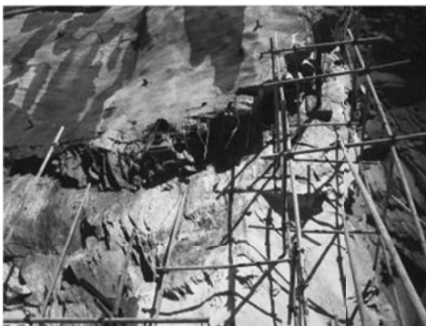
Figure 7.184 Rock mass collapse near fault F_{16} .
