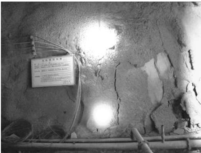
Figure 7.214 Sprayed concrete cracks near #1 construction tunnel entrance.
