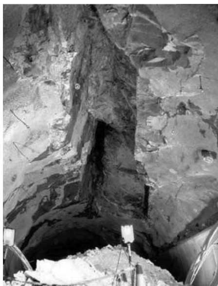
Figure 2.5 Hanekleiv Road Tunnel, Norway, where a section of tunnel caved in 10–11 years after excavation having unfavourable rock geometry with joints almost parallel to the tunnel axis.
