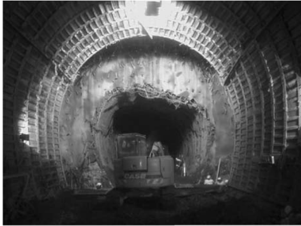
Figure 6.37 Saint Martin La Porte access adit at chainage 1325 m before removing the tunnel cross-section (Barla et al., 2011).
