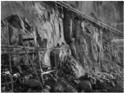
Figure A22 Collapse at fault F16 fracture zone.
