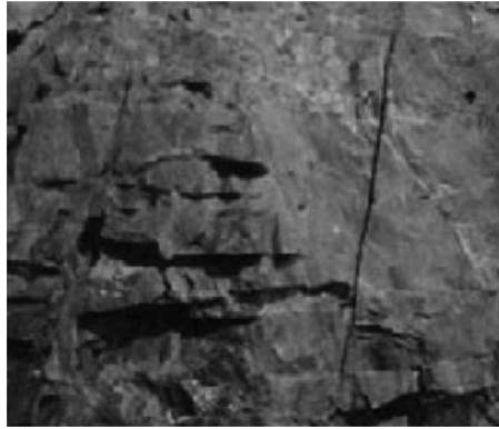
Figure A18 Splitting crack at the transformer chamber upstream sidewall.
