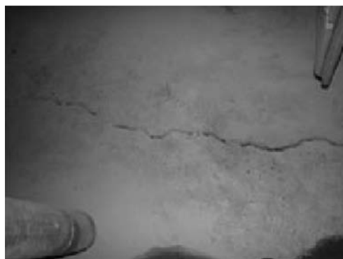
Figure A17 Circumferential cracks at 1# construction tunnel invert.
