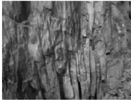
Figure A26 Bedding plane splitting in the sidewall.
