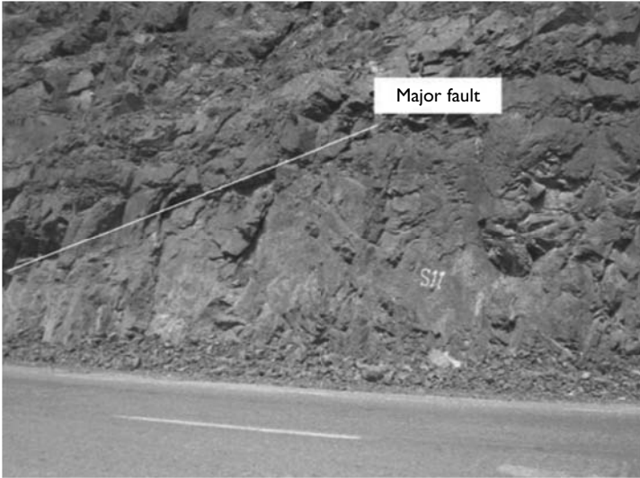
Figure 3.38 Nature of the rock mass along the Khosh-Yeylagh main road in Iran (from KhaloKakaie & Zare Naghadehi, 2012).
