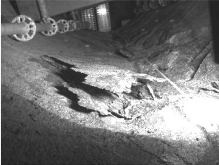
Figure 5.20 Rock spalling as a result of locally increasing the in situ rock stresses around a simulated deposition hole at the Äspö HRL (Andersson, 2007).
