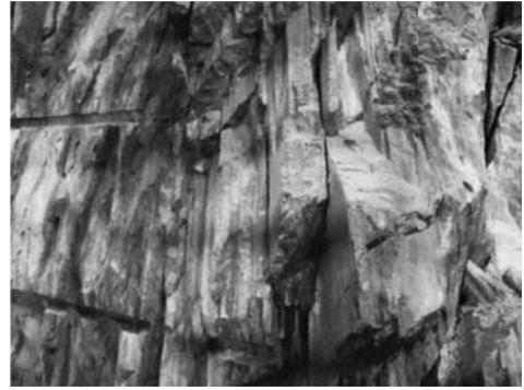
Figure 7.176 Rock cracking at cavern intersection.
