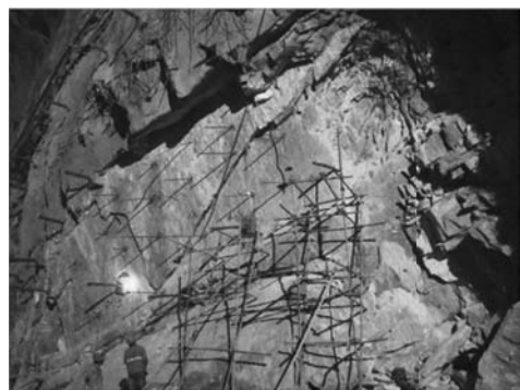
Figure 7.185 Overbreak near fault F_{21} .
