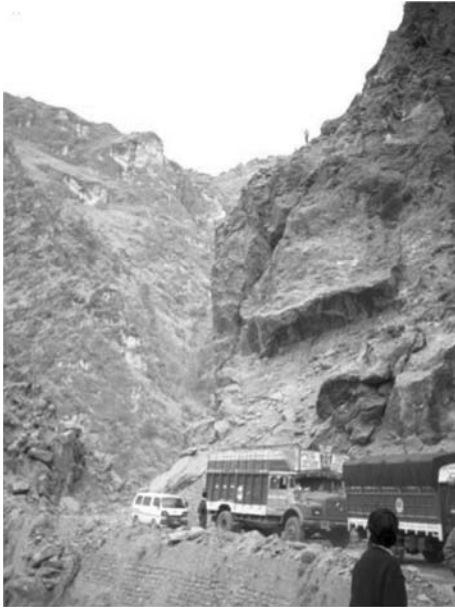
Exposure 1. Fractured and weathered roadside rock slope, India
