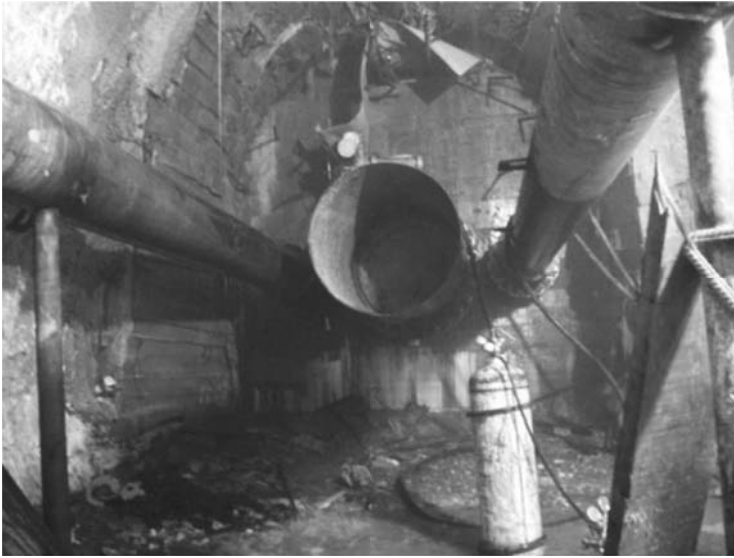
Figure 6.78 Treatment for the high pressure flow point in the lower sidewall near AK14+760 in Access Tunnel #A (HydroChina Huadong Engineering Corporation, 2005).
