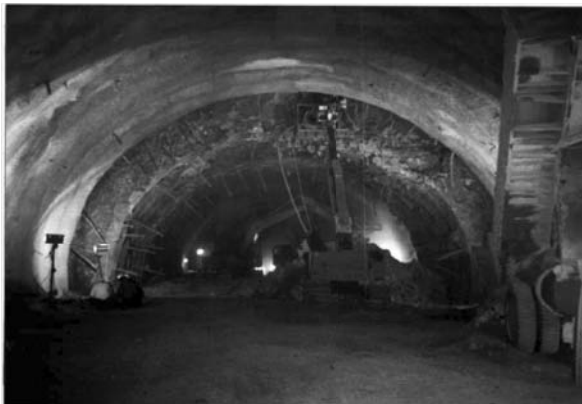
Figure 6.36 Re-mining the perimeter of the 16 m span Mucha tunnel in Taiwan after severe squeezing in a fault zone. Photograph reproduced with permission from Sinotech Engineering Consultants Inc., Taipei (Hoek, 2001).
