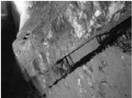
Figure A23 Fault sliding at draft tube gate chamber.
