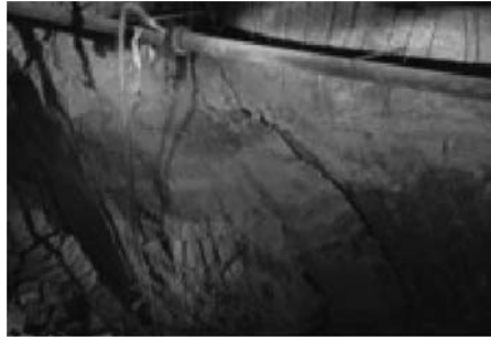
Figure A27 Joint loosening and opening in the transformer chamber sidewall.
