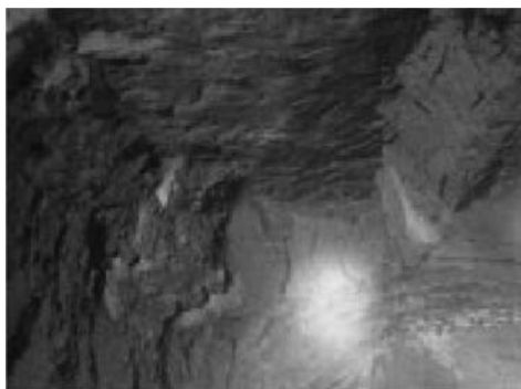
Figure A16 Rock block falling at vault of draft tube gate chamber.
