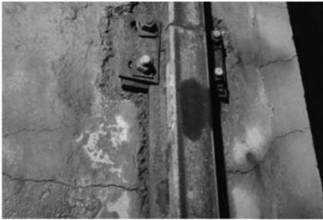
Figure A30 Cracks at the top of the upstream rock anchor beam.
