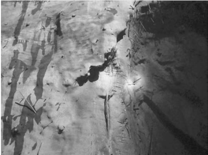
Figure 7.215 Rock block collapse near #3 bus tunnel entrance.
