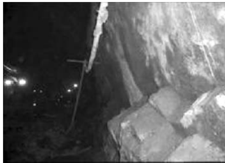
Figure A1 Tilting failure of powerhouse upstream sidewall.
