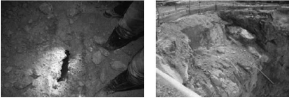
Figure A12 Surrounding rock failure process at the 3# pit sidewall.
