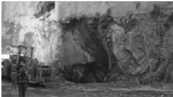
Figure A19 Collapse at the intersection of high pressure pipe and sidewall.
