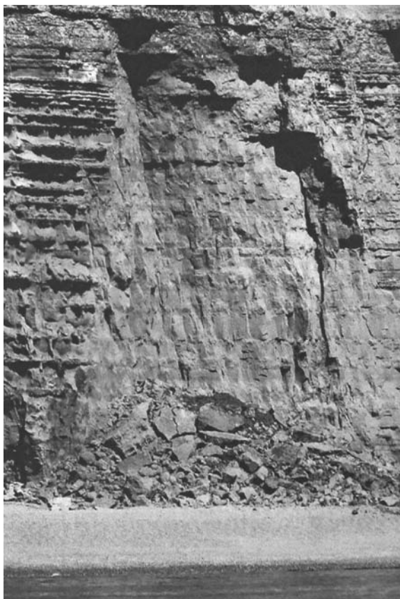
Figure 2.12 Beach cliff fall in horizontal sandstone strata with alternating weak and soft layers, plus sub-vertical fractures. Failure is caused by undercutting erosion and then sliding on the sub-vertical planar fractures (Jurassic Bridport Sands, UK).
