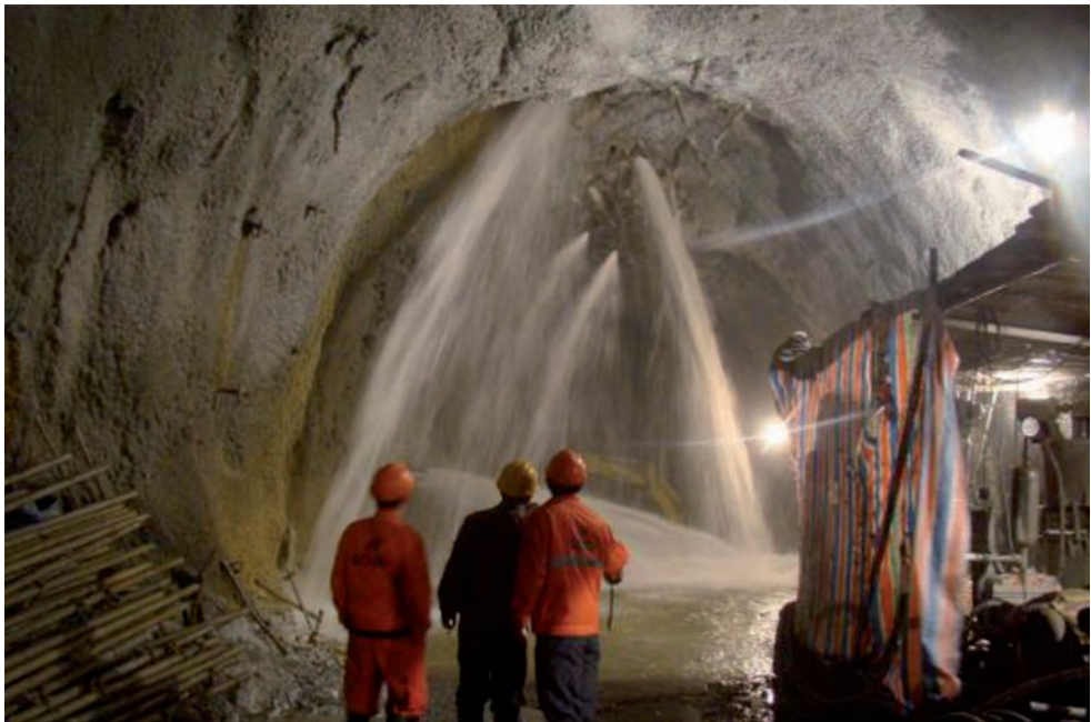
Figure 6.79 High pressure flow point near the tunnel crown at chainage AK10+612 in Access Tunnel #A: (a) before treatment.
