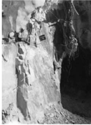
Figure A20 Collapse at 3# bus tunnel intersection.
