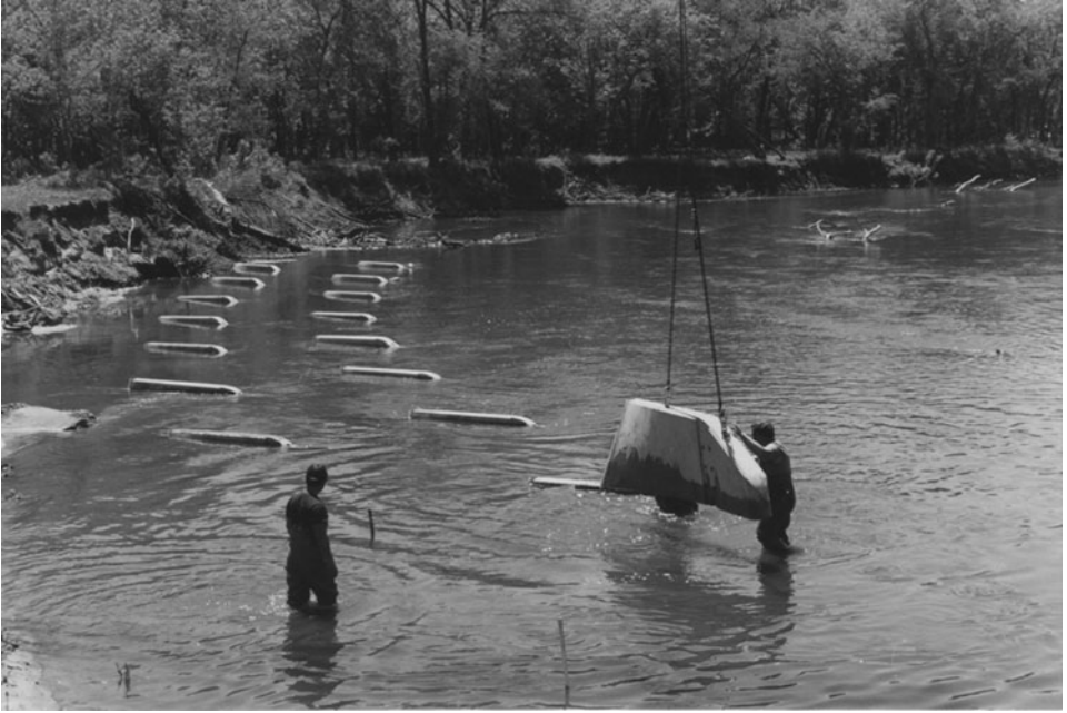
Figure 5-9. Vane is lowered in place on top of pile, summer, 1988. Source: Odgaard and Abad (2007), ASCE.
