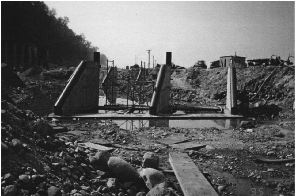
Figure 5-63. Installation of vane system. View downstream, showing intake on the left, the cofferdam on the right, and the slab with a set of three vanes in the middle. Courtesy of J. Oosterman, DHV Consulting Engineers.
