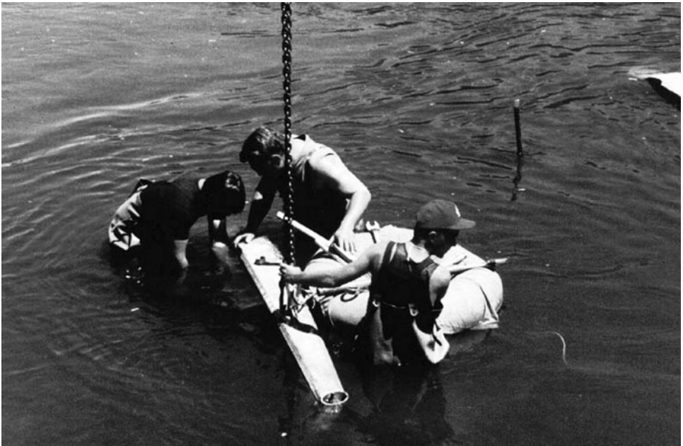
Figure 5-10. Vane is connected to pile, summer, 1988. Courtesy of Robert DeWitt, River Engineering International.
