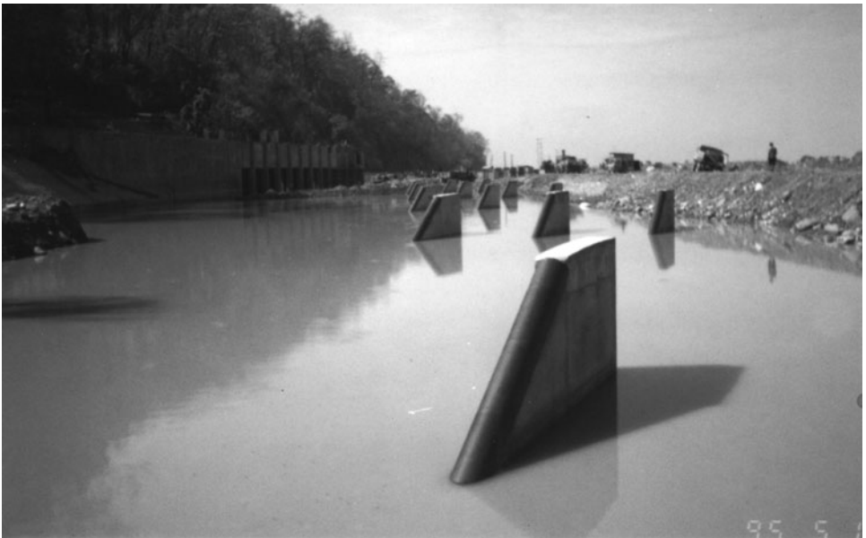
Figure 5-64. View downstream of completed vane installation in Kosi River. The intake is on the left and the cofferdam on the right. Courtesy of J. Oosterman, DHV Consulting Engineers.
