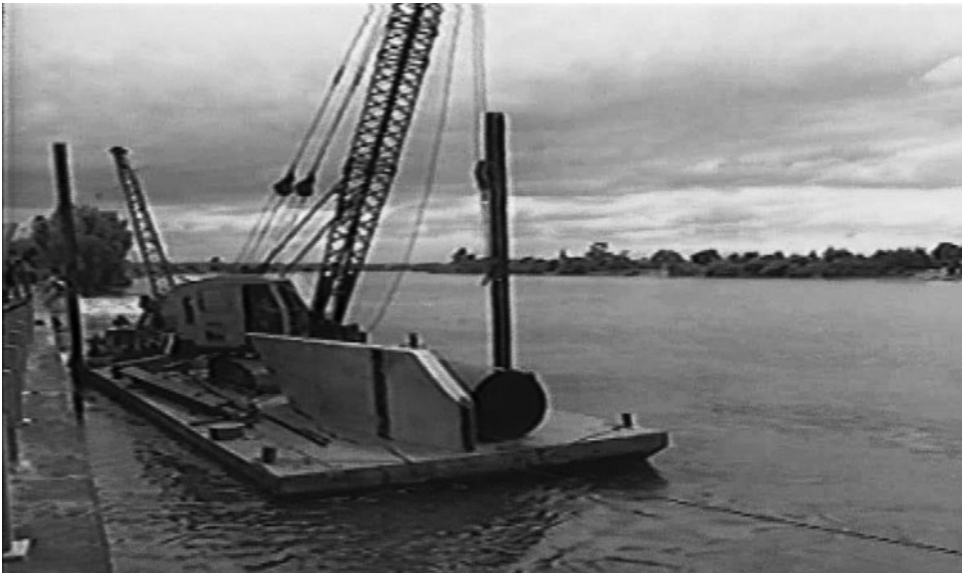
Figure 5-43. Huntly vane, and pipe and pipe follower on barge outside the intake. Source: Electricity Corporation of New Zealand (1993), with permission from Genesis Energy.
