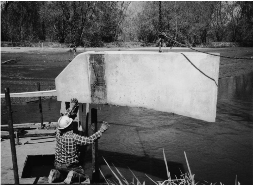
Figure 6-7. Vane installation in Clear Creek, Iowa. The vane is slipped over an H-pile that fits inside a circular cut-out of the vane. Courtesy of Robert DeWitt, River Engineering International.
