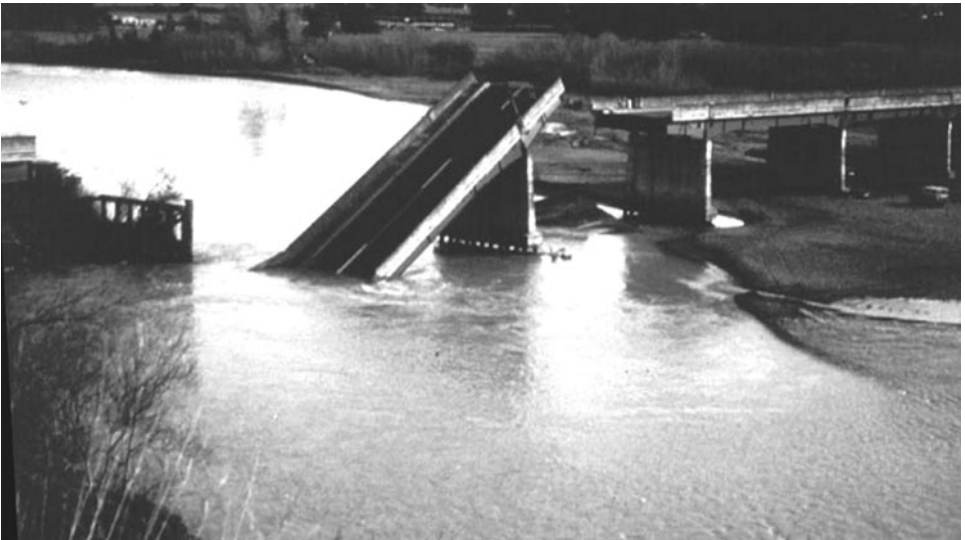
Figure 1-2. Abutment scour at Bulls Bridge over Rangitikei River, New Zealand. Source: Raudkivi and Ettema (1985), ASCE.
