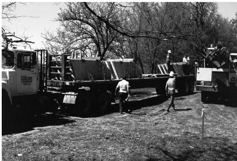
Figure 5-7. Delivery of vanes to the Wapsipinicon site, summer, 1988. Courtesy of Robert DeWitt, River Engineering International.
