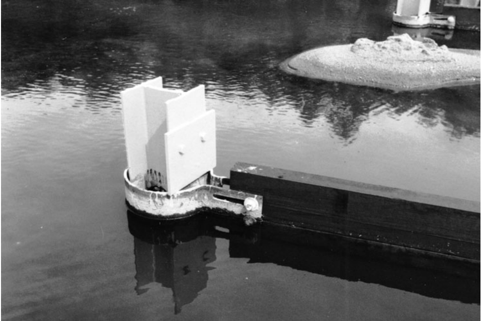
Figure 6-5. Vanes in East Nishnabotna River, Iowa consist of vertical planks supported by H-piles. They are prevented from floating by anchor plates on the flanges of the H-piles.
