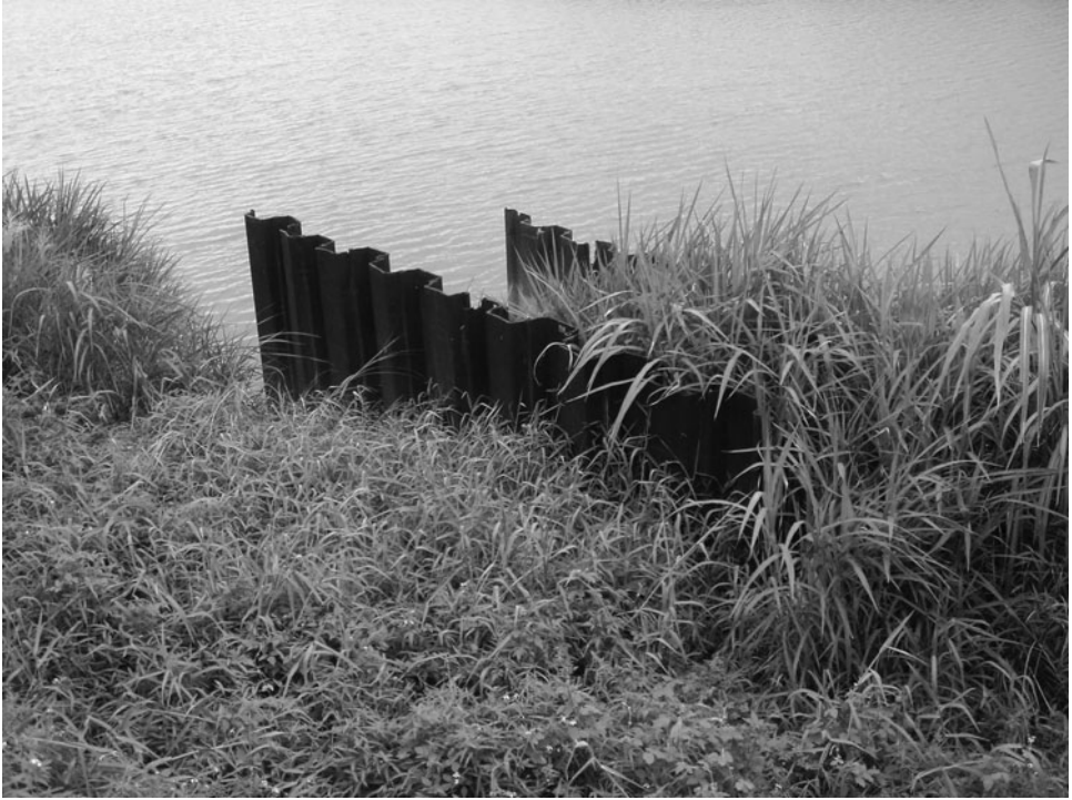
Figure 5-21. Close-up of vane array in the Maoerding bend, one year after installation, at extreme low flow.
