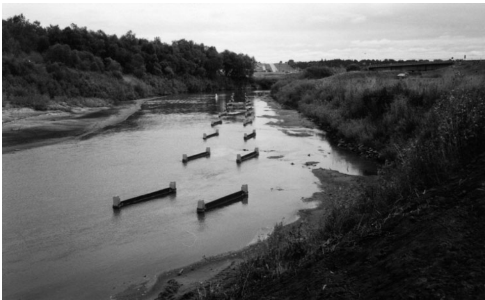
Figure 1-6. Submerged vanes (early version) in East Nishnabotna River, Iowa, protecting stream bank against erosion. View is downstream at extreme low flow, showing vane-induced sediment deposition along right bank. The sediment deposits provide natural toe protection at the bank.
