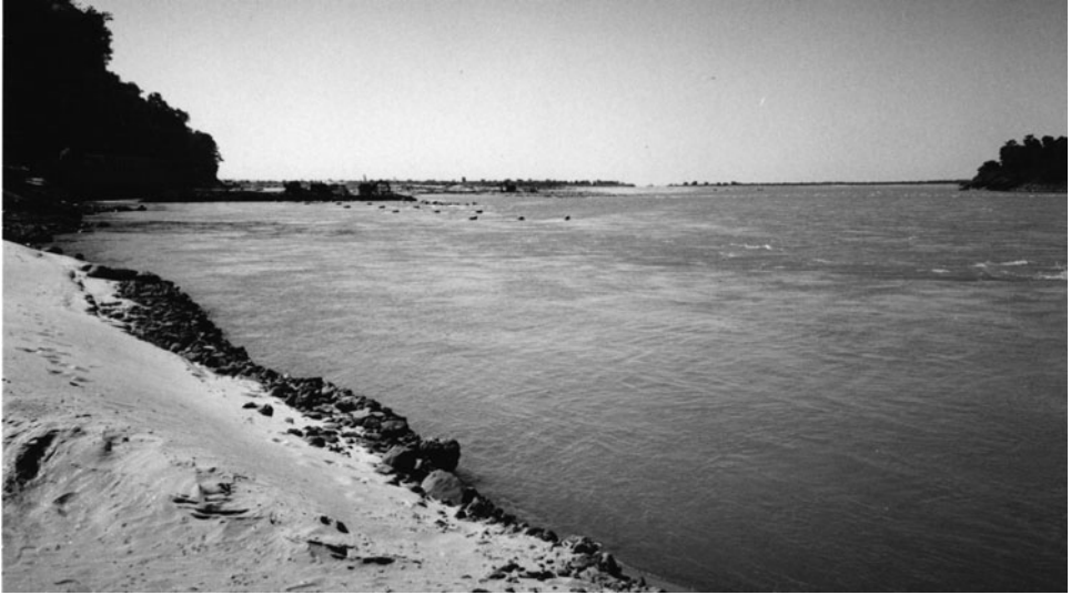
Figure 5-65. Vane installation in Kosi River. View downstream shortly after completion, at extreme low flow. Most of the cofferdam has been removed. At elevation 109.5 m, the tops of the downstream vanes are above the water surface. Courtesy of J. Oosterman, DHV Consulting Engineers.
