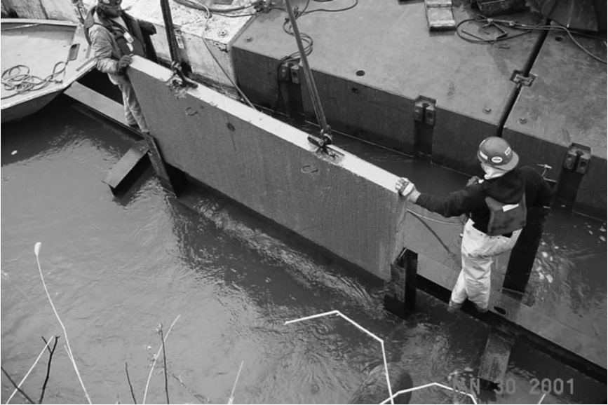
Figure 5-54. Precast concrete vane panels being placed between H-pile supports. Placement guides extend temporarily above the H-columns. Source: Michell et al. (2006), ASCE.
