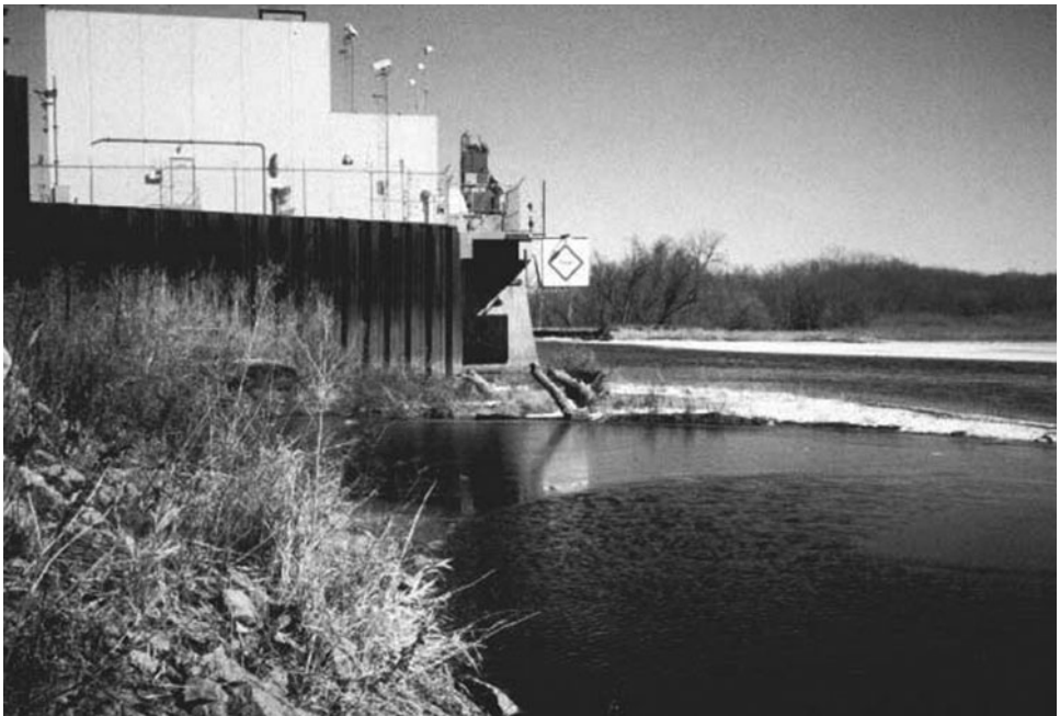
Figure 5-30. View upstream toward the DAEC intake structure, showing a sandbar in front of part of the intake.
