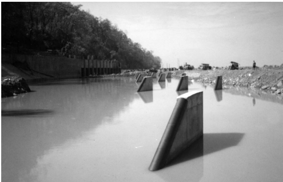
Figure 1-5. Submerged vanes being installed at water intake on Kosi River, Nepal. View is downstream and inside of coffer dam (right). The vane system will prevent sediment from being entrained into the intake (left). Courtesy of J. Oosterman, DHV Consulting Engineers.
