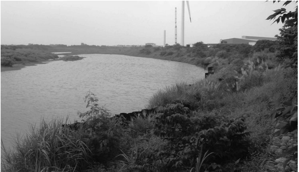
Figure 5-20. Downstream view of vane installation in the Maoerding bend, one year after installation, at extreme low flow.
