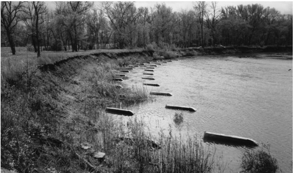
Figure 5-11. Wapsipinicon River bend at low flow, May 10, 1990, about two years after installation of vanes. Source: Odgaard and Abad (2007), ASCE.
