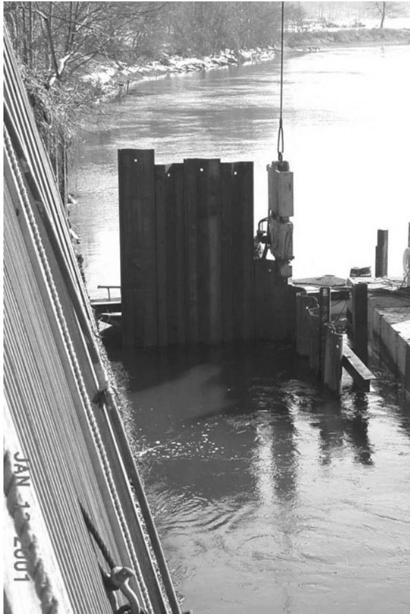
Figure 5-53. Sheet-pile being driven into the bed to form a skimming wall. Source: Michell et al. (2006), ASCE.
