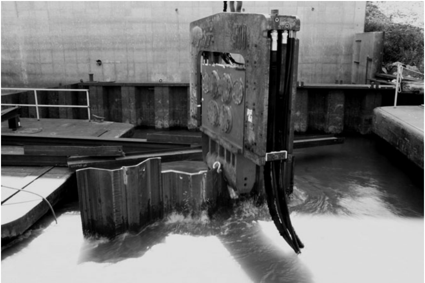
Figure 6-3. Vane installation at Cooper Station, Missouri River. Following alignment along the guide and minimum penetration into the bed (Fig. 6-2), all sheet-piles are driven to final elevation using a vibratory driver. View toward face of the intake. Courtesy of Rhoël M. Tierra, Nebraska Public Power District.
