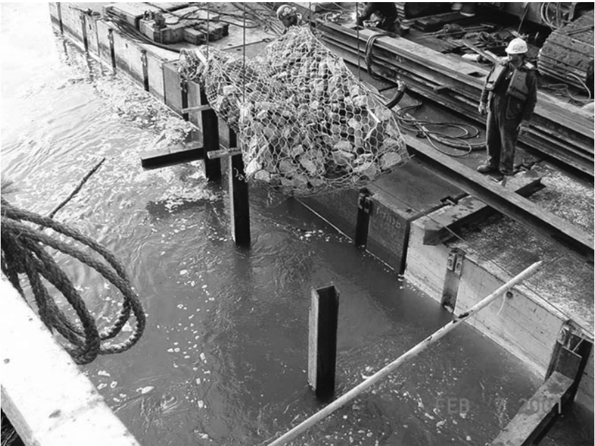
Figure 5-55. Mat protection being placed at the base of the vanes. Source: Michell et al. (2006), ASCE.
