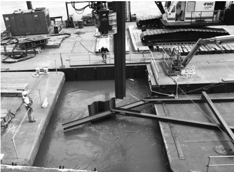
Figure 6-2. Vane installation at Cooper Station, Missouri River. Sheet-pile vanes are being installed along the guide for vane alignment. Flow is from left to right. Face of intake is at bottom of photo. Courtesy of Rhoël M. Tierra, Nebraska Public Power District.
