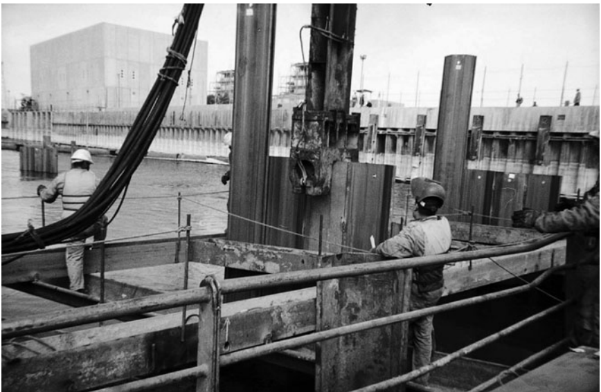
Figure 6-4. Vane installation at Kuraimat Power Station, the Nile River, Egypt, 2007. Photo shows sheet-piles being driven in a template that controls vane orientation. Intake is in the background of the photo. Courtesy of Adnan M. Alsaffar.
