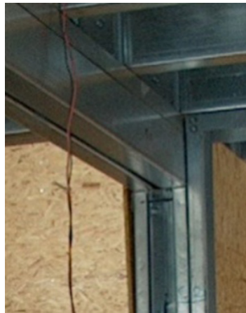
Figure 8.67 – Example of web stiffener and double joists at Constantin House (SP024a-EN-EU, AccessSteel 2006)
