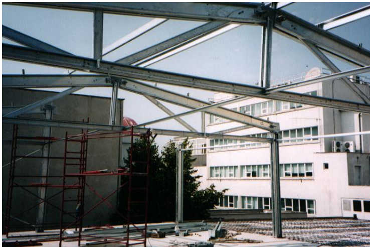
Figure 1.31 – Trusses made of double built-up channel section for a penthouse structure (Alcatel Timisoara, Romania)
