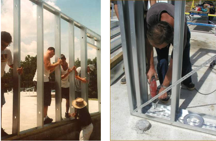
Figure 8.19 – Phase III: Walls are assembled on the floor and then lifted up in vertical position
