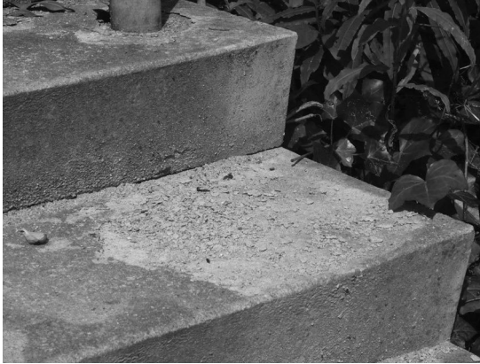
Figure 2.38 Scaling of concrete steps.
