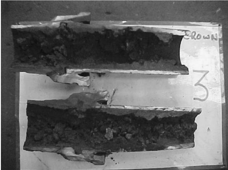
FIGURE 4.31 A sample of internal tuberculation in unlined cast iron potable water pipe. (Source: 3M Corrosion Protection Products.)
