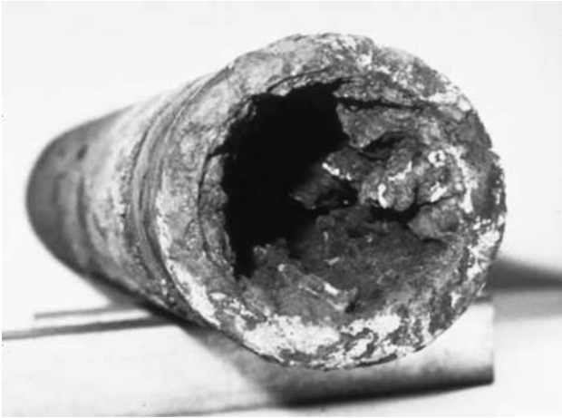
FIGURE 3.1 Excessive tuberculation in water pipes. (Source: 3M Water Infrastructure.)
