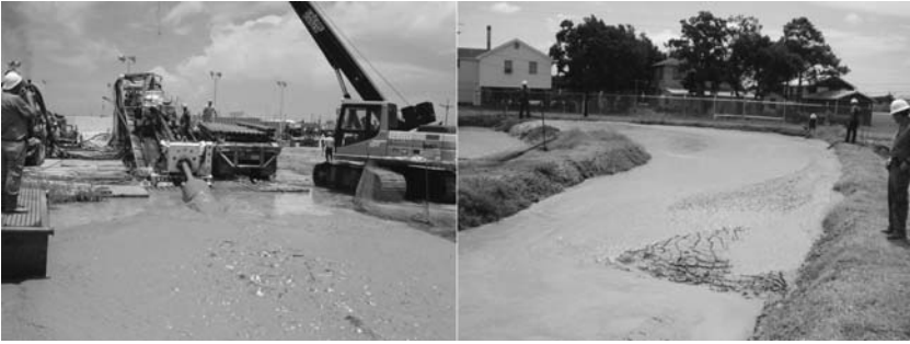
FIGURE 5.9 Drilling fluid disposal can be a major operation in Maxi-HDD operations. (Source: Trenchless Engineering Corporation.)
