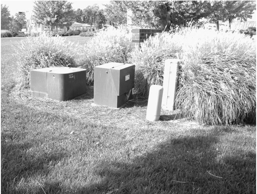
Figure 5-2. Utilities. Contact all utility companies early in the project planning phase and request utility layout plans. Proper scheduling of utility companies for installation is critical to meeting the overall project schedule.
