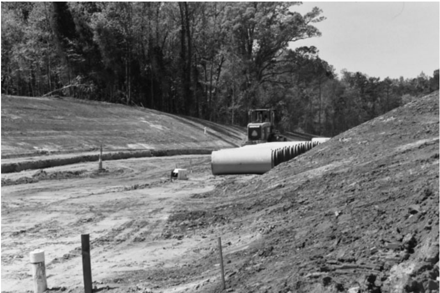
Figure 9-1. Earthwork. Use site contours to minimize cuts and fills is the goal of the engineering design. Contractors are using GPS guided equipment to undertake earthwork operations.
