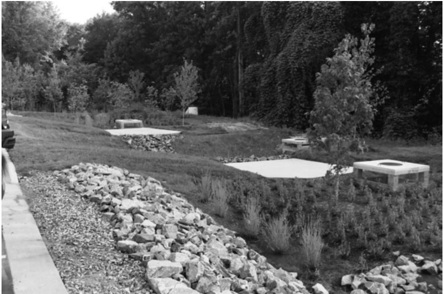
Figure 12-4. Extended Detention Facility. In this photo, the facility consists of a forebay, rain garden and an extended detention facility. Stormwater runoff is controlled in an extended detention facility for 48 hours prior to being discharged.
