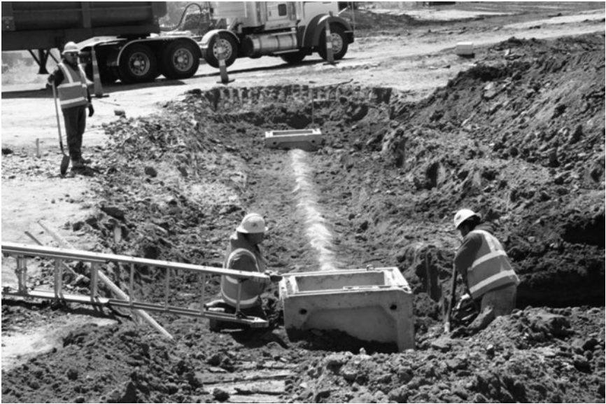
Figure 7-3. Engineering Design. Land development projects require a civil engineering design discipline to reduce site costs and for regulatory compliance. Source: David E. Johnson, P.E., P.P.
