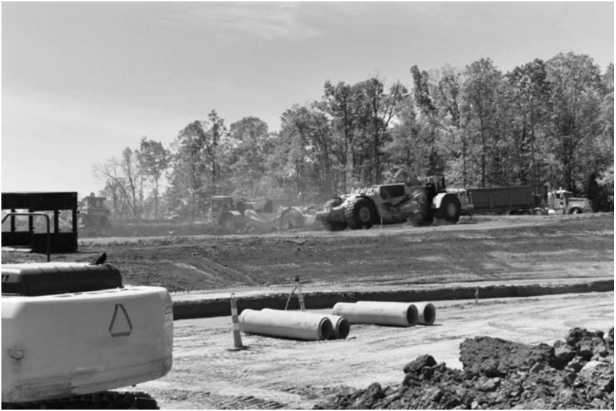
Figure 15-1. Field Management. Developer personnel or representatives supervise construction activities and approve contractor invoices in accordance with the negotiated contract. Typically, developers will not pay the contractor for material delivered and stored on site.
