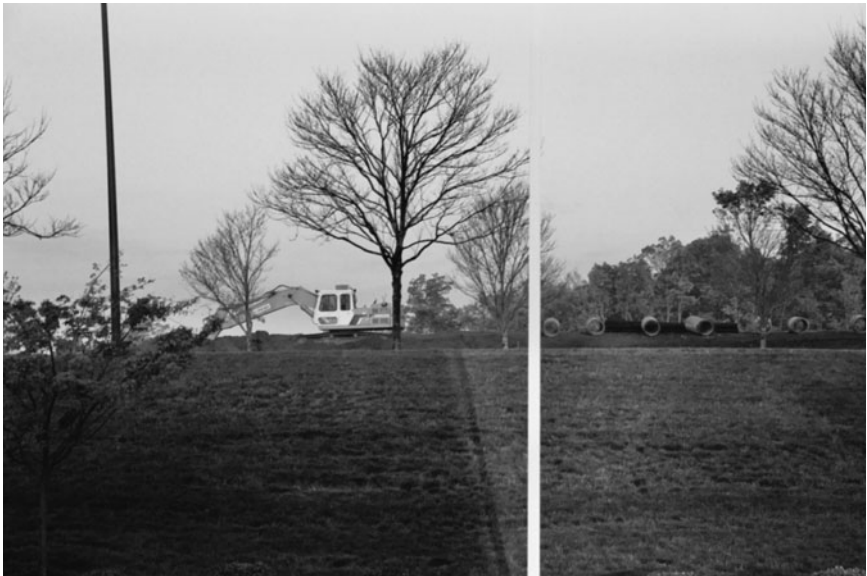
Figure 16-2. Drainage Facilities. Erosion control and stormwater management facilities must be installed and operate properly to adequately control runoff during the construction process. Erosion and sediment are visible and indicative of the lack of quality control.
