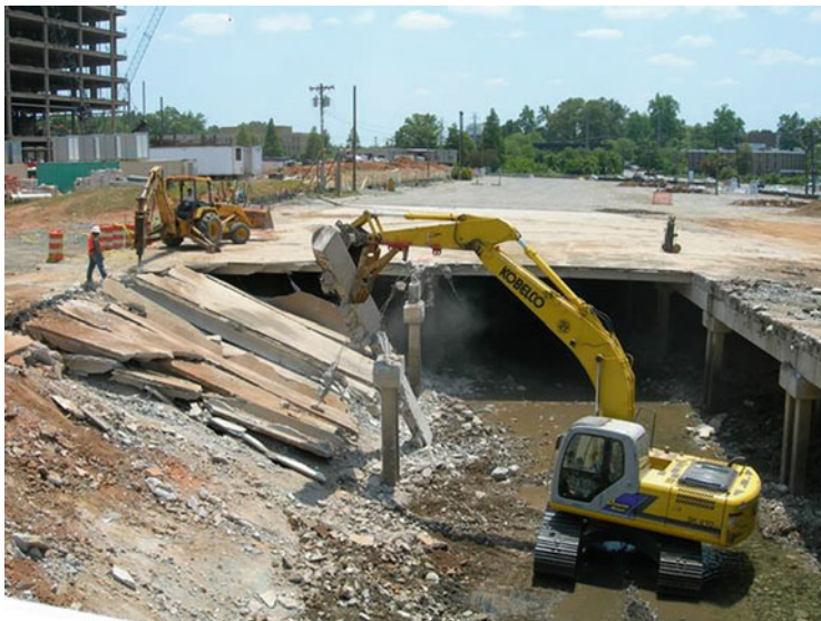
Fig. 11 Former Midtown Mall parking deck during demolition, Jay Higginbotham, Mecklenburg County Asset and Facility Management (Image courtesy of Crystal Taylor, P.E., Charlotte–Mecklenburg Storm Water Services, 2007)
