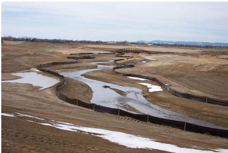
Fig. 16 Westerly Creek at Stapleton in early channel construction (Image courtesy of Jane Kopperl, Matrix Design Group (EDAW) 2002)
